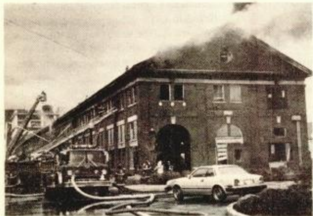
CONSTRUCTION of the Anchorage Apartments at Building 103 in the Charlestown Navy Yard will be delayed as a result of a smoky six alarm fire on Wednesday, March 13, 1985. The blaze caused extensive damage to the third floor and roof of the former sheet metal building.
