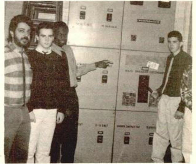
FACULTY MEMBER Robert Domenico (left), of the Electricity technology department at Don Bosco Technical High School in Boston, with students (from second left) Shawn M. Branco of Somerville, Gregory Ferdinand of Cambridge and Daniel F. Wallace of 11 Mt. Vernon Street, Charlestown, operate a 500 amp disconnect on a switchboard. Students in the program either go on to college to pursue engineering technology or to jobs in the electrical industry as apprentices.
