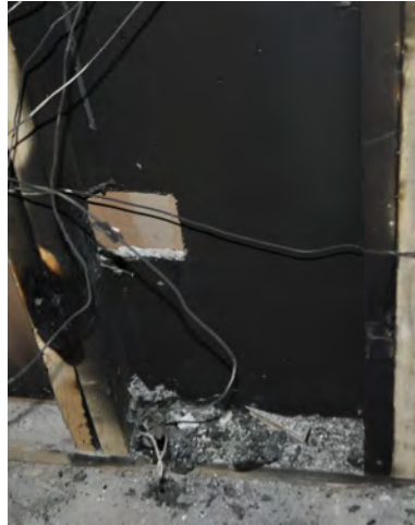
(b) Double Switch & Outlet Post Fire Rear
