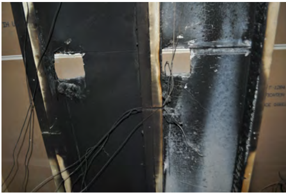
(c) Double Switch & Outlet Rear Middle
