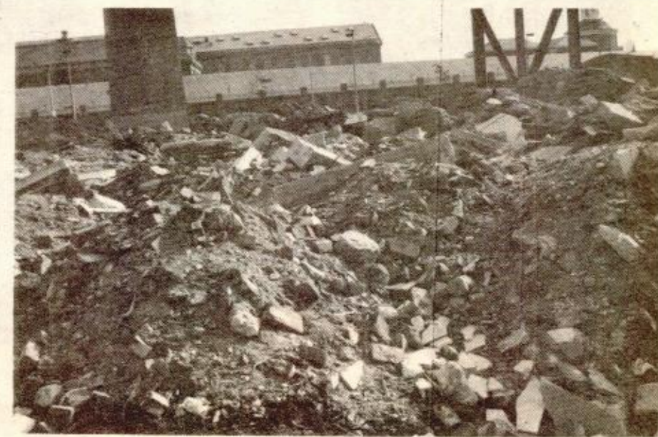
DANGEROUS AND UNSIGHTLY mounds of debris were visible on Sunday, January 24th in this view from Hunter Street looking towards the Charlestown Navy Yard. This site has been the subject of numerous complaints from residents.
