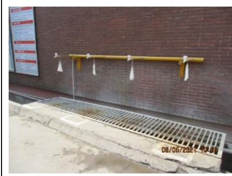
COVID19: Hand wash facility
