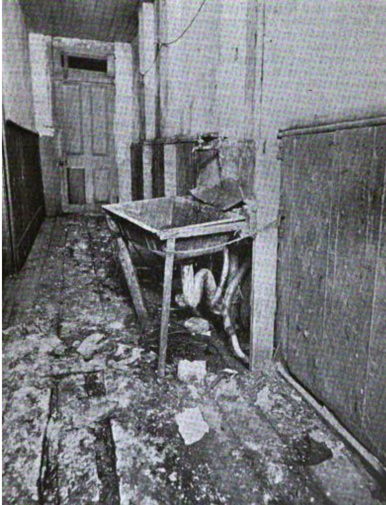
Photo 1.7: Public hall and sink. Sink supported only by string and flimsy wooden props. Hall floor covered with fecal matter and sewage. (1903)
