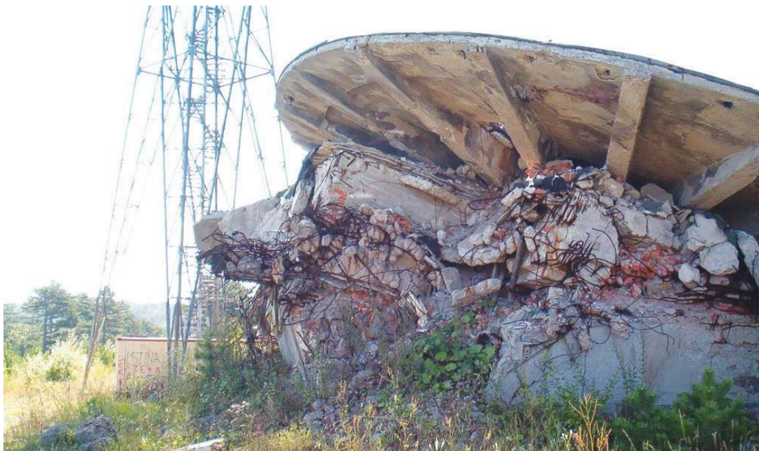
Picture 28. Destroyed repeater “Kraljica” on Ozren Mountain
