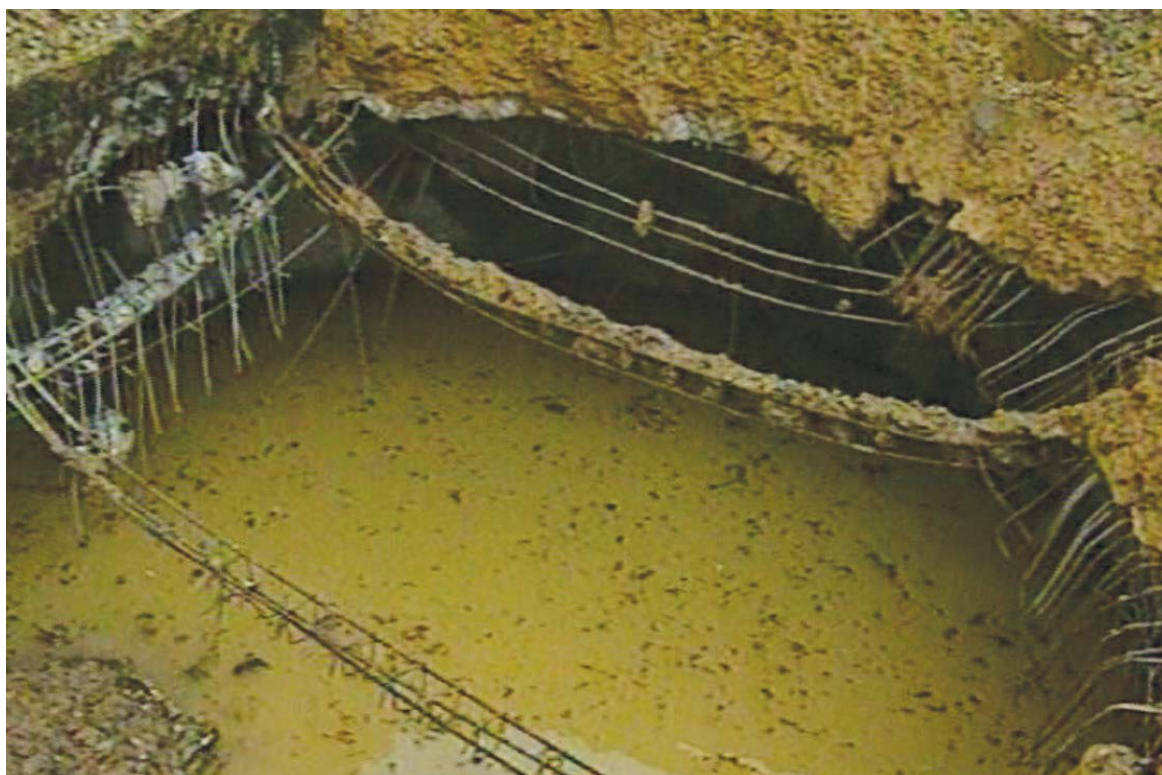
Picture 49. Destroyed water reservoir in Lukavica
