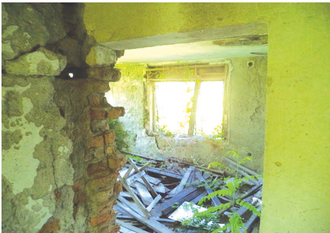
Picture 39. Inside the destroyed house of the Goranovic family
