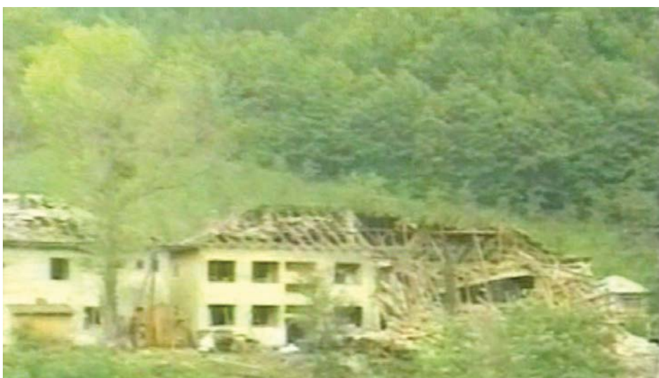
Picture 9. Destroyed residential building in Srbinje
