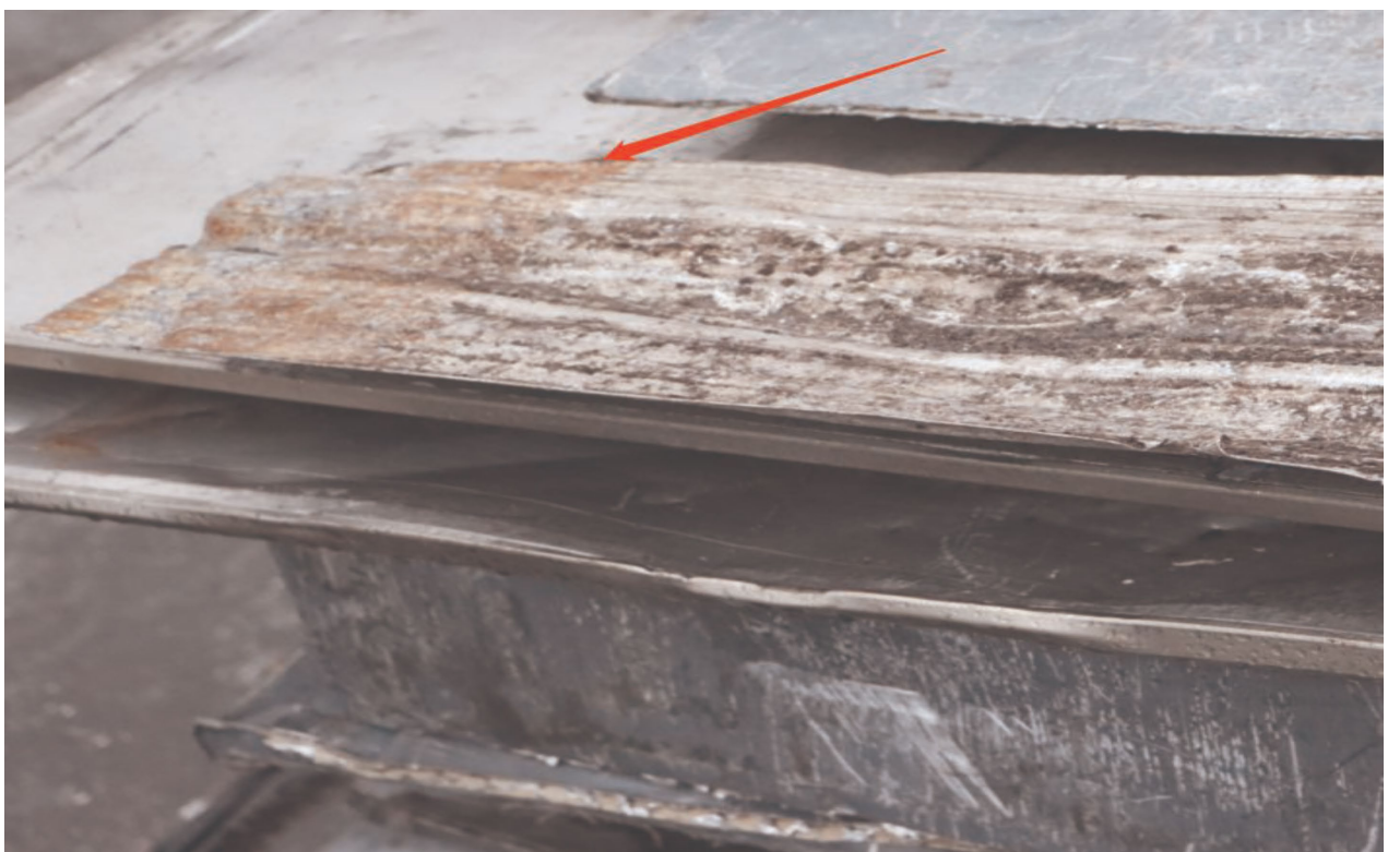
Figure A.14 Mud, sand and pollution corrosion products on the surface of aluminum plate
