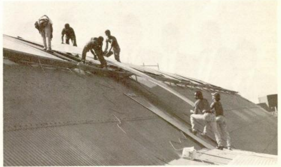
WORKMEN replace the roof at the Emmons-Horrigan-O'Neil Skating Rink with the $350,000 job expected to be completed by next Monday's opening.
