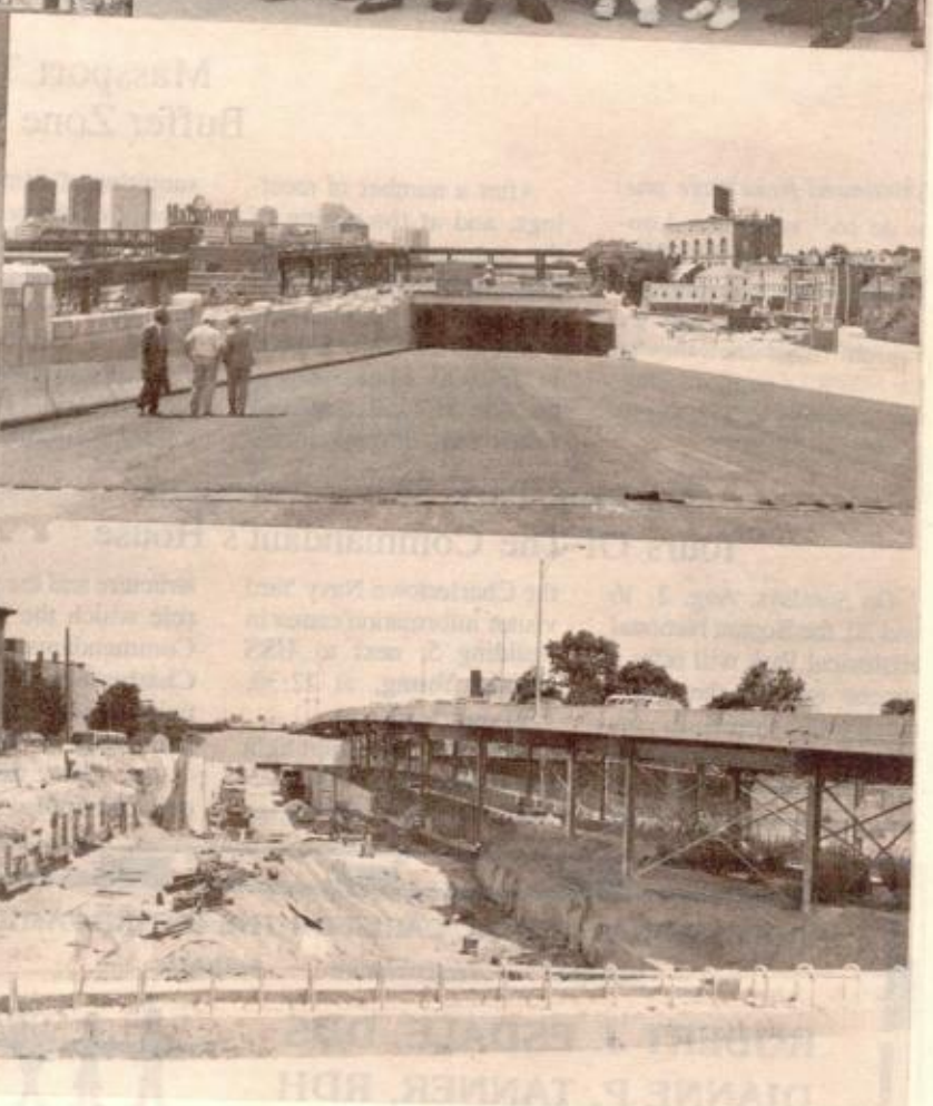
of the Tobin Bridge tunnel connection which is near completion. Lowney Way can be seen on the left with Chelsea Street shown beneath the temporary bridge off-ramp on the right.
