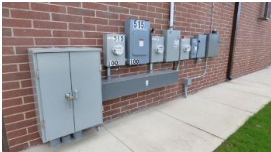
The service entrance is in the rear, on site drop down transformer noted. Each suite in individually metered.
