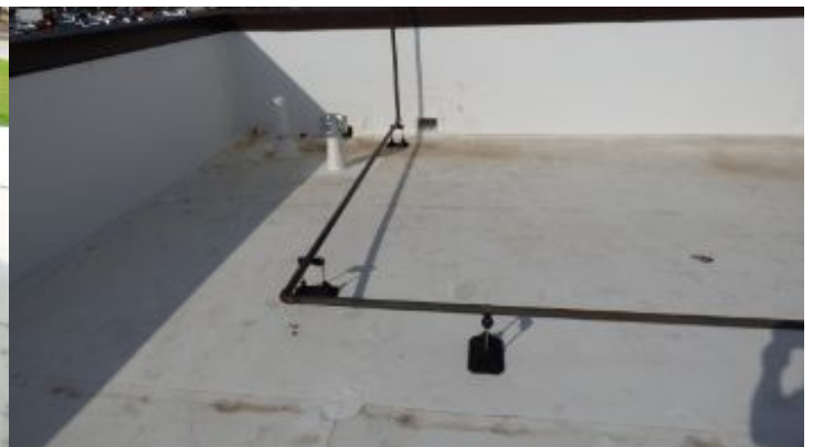
Gas lines at roof top
