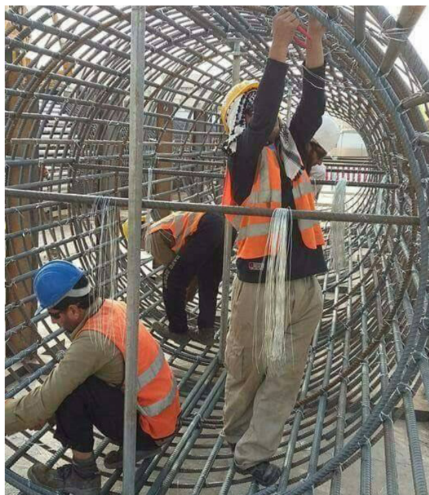
Workers on Lusail Stadium, where the final of the FIFA World Cup Qatar 2022 will be played, described experiencing tension and exhaustion because of their working and living conditions. © Equidem 2022
