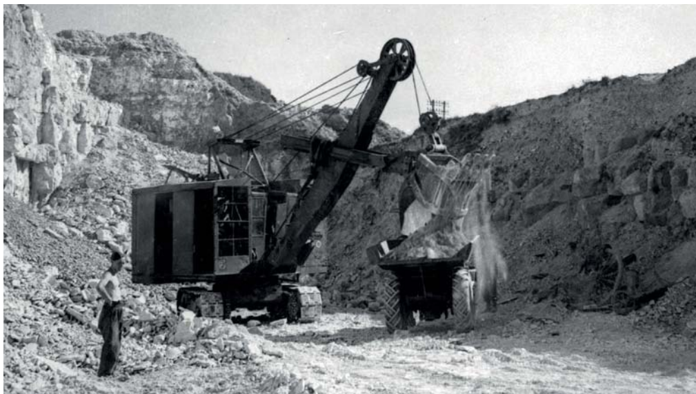
Above: A mechanical excavator operated by 4854 Quarrying Flight at a quarry between Carpiquet and Caen in Normandy, releases stone for the repair and construction of runways and airfields. RAF (AHB)/© UK MoD Crown Copyright 2014
