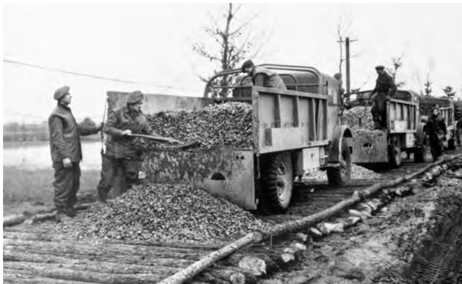
ABOVE: Using logs and gravel, Royal Engineers work to improve the roads that British units will traverse during the upcoming Operation Veritable. BELOW: M4 Sherman medium tanks of the 15th Scottish Division, Argyll and Sutherland Highlanders assemble at their jumping-off point for the beginning of Operation Veritable.
