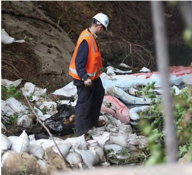
RBC oil spill clean-up
