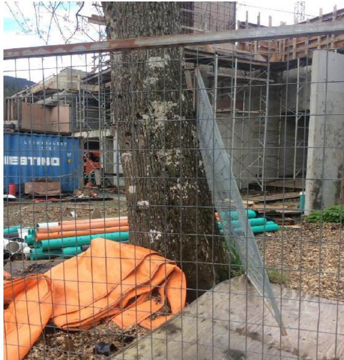
Figure 5. Construction piled against one of the large oaks on Lillooet Road; no tree protection present.
