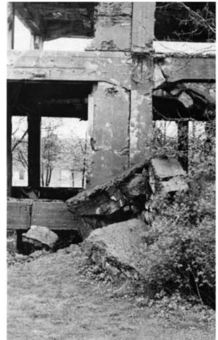
Forster and Kleikamp look on. Right: Unfortunately that was the wing which has since been demolished but this is exactly the same angle today.
