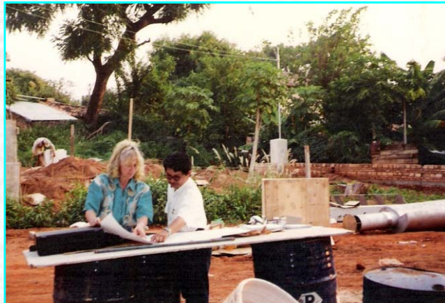
Engeneering Lambaré> Treatment Plants
