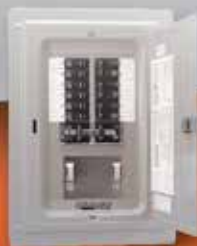
CIRCUIT PANEL UPGRADE
