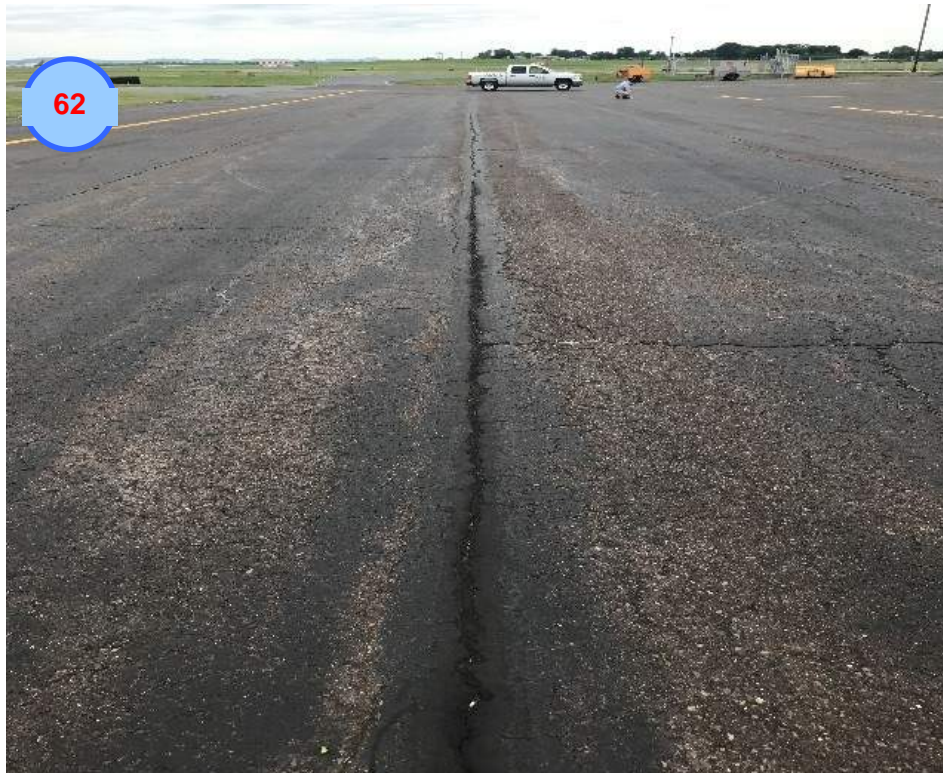
Medium Severity Longitudinal Cracking and Weathering
