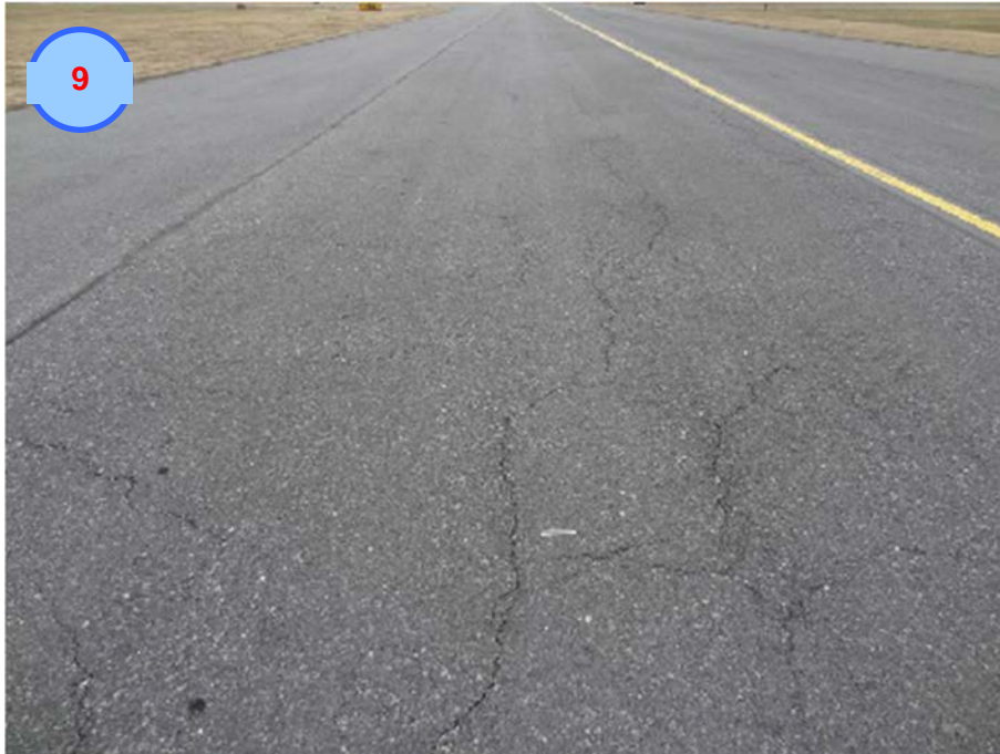
Low severity Longitudinal Cracking Western Portion
