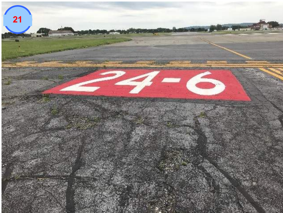
Alligator Cracking and Rutting
