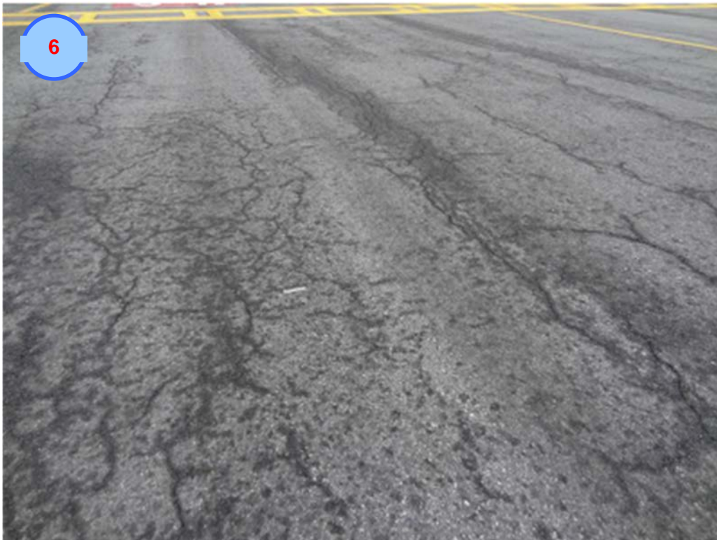
Medium Severity Block Cracking
