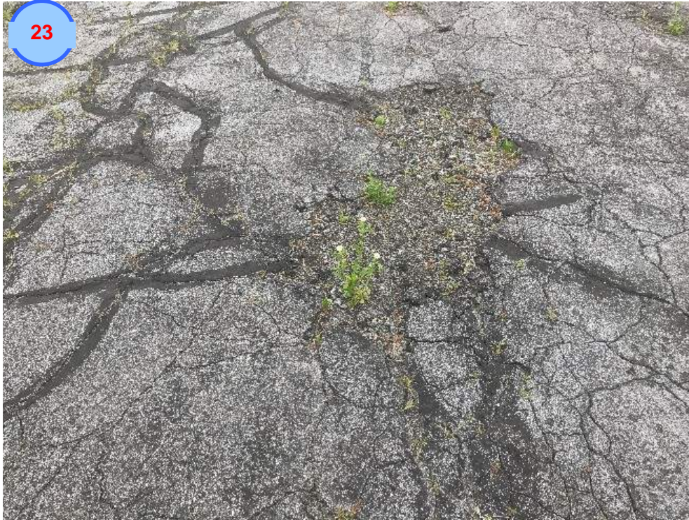
Medium Severity Alligator Cracking, Raveling
