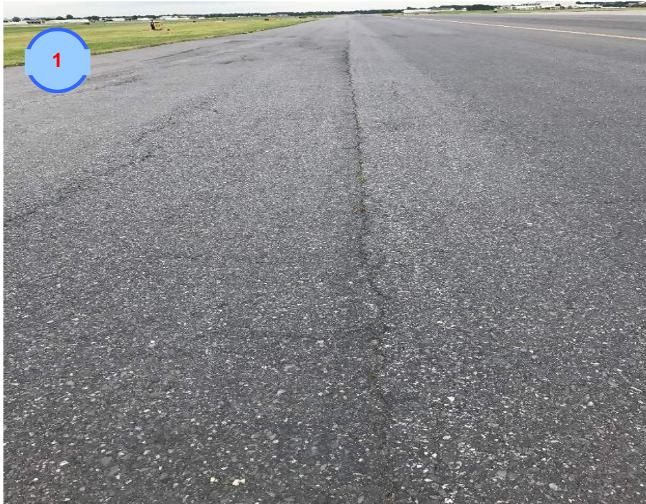
Low Severity Longitudinal Cracking
