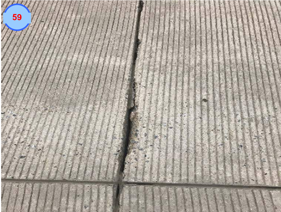
Joint Seal Damage and Spalling PCC Apron
