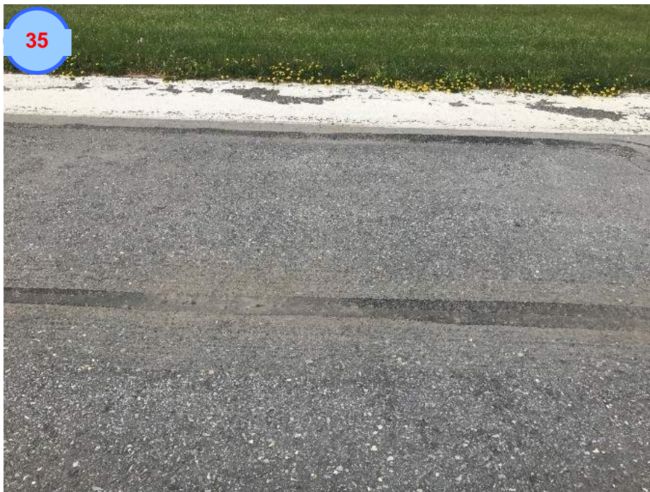
Low Severity Weathering and Longitudinal Cracking
