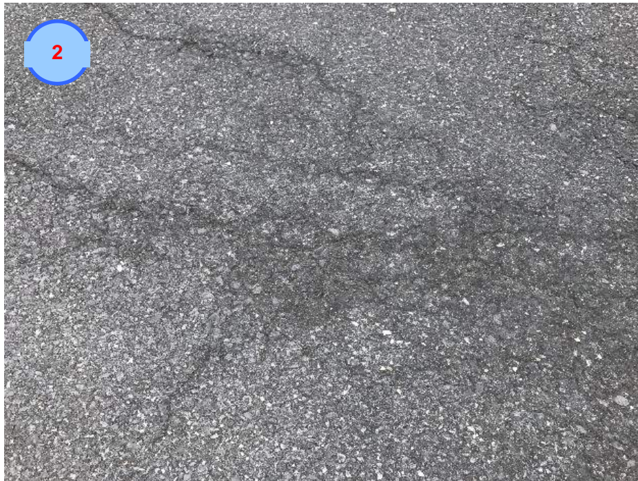
Low Severity Longitudinal Cracking, Weathering, and Raveling
