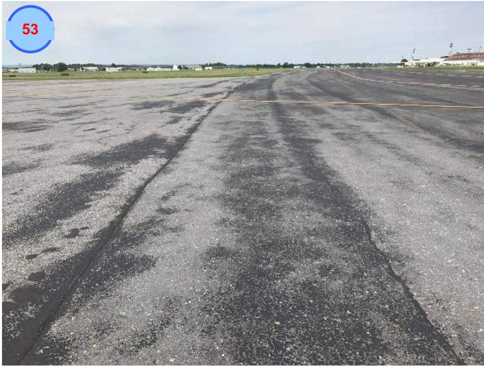
Longitudinal Cracking, Bleeding, and Weathering West Section
