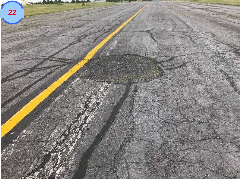
Medium Severity Alligator Cracking, Depression, Rutting, and Patching
