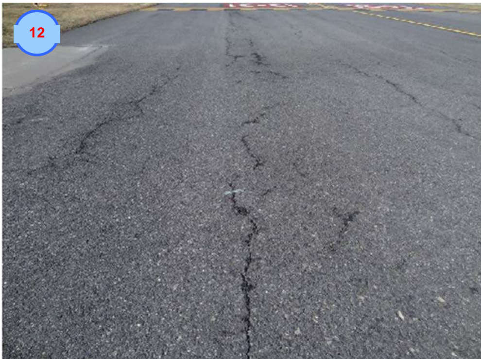
Cracking and Weathering
