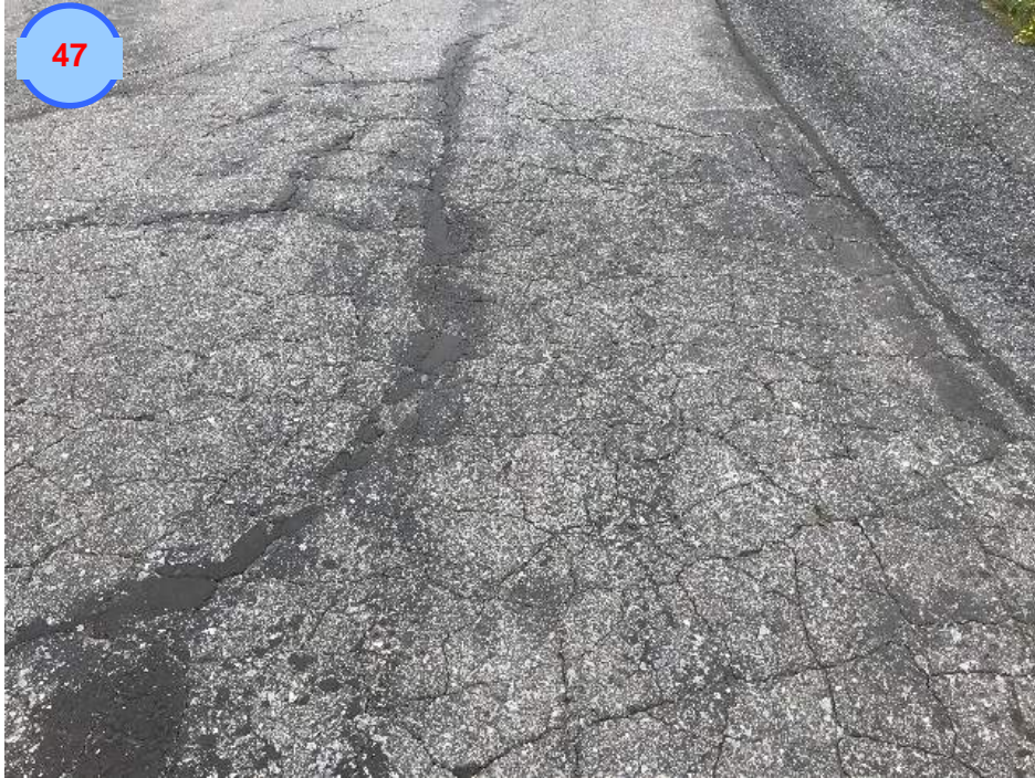
Medium Severity Alligator Cracking, Bleeding, and Weathering
