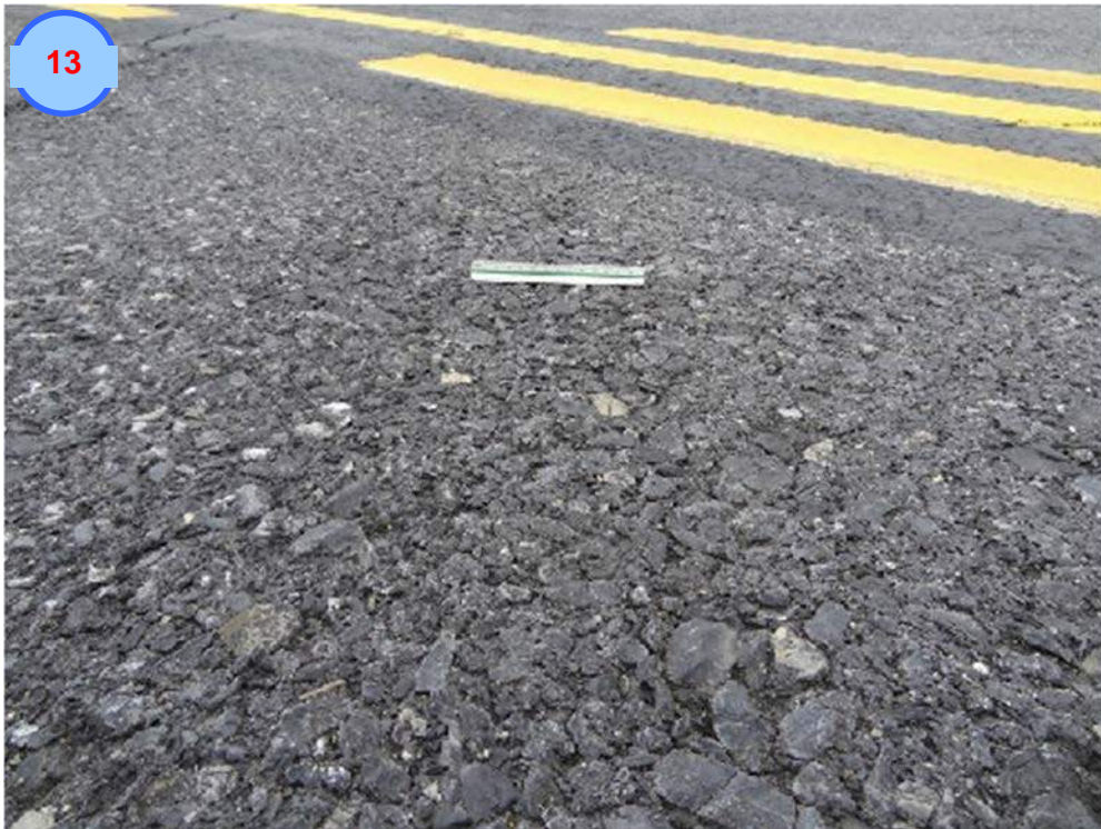
Medium Severity Weathering
