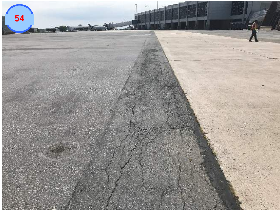
Alligator Cracking and Raveling at AC/PCC Transitional Pavement
