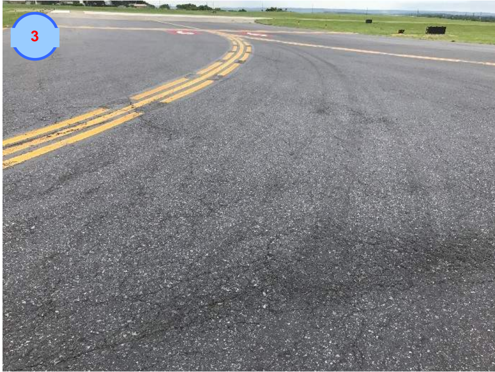
Low severity Weathering and Low Severity Alligator Cracking
