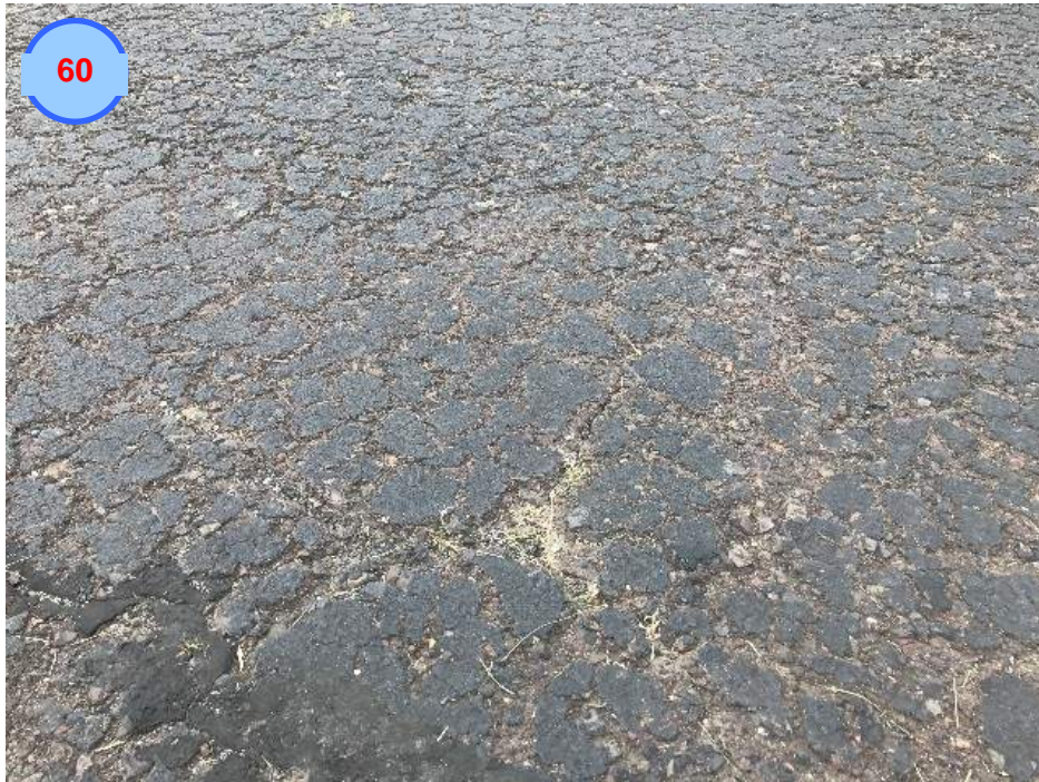
High Severity Weathering and Raveling
