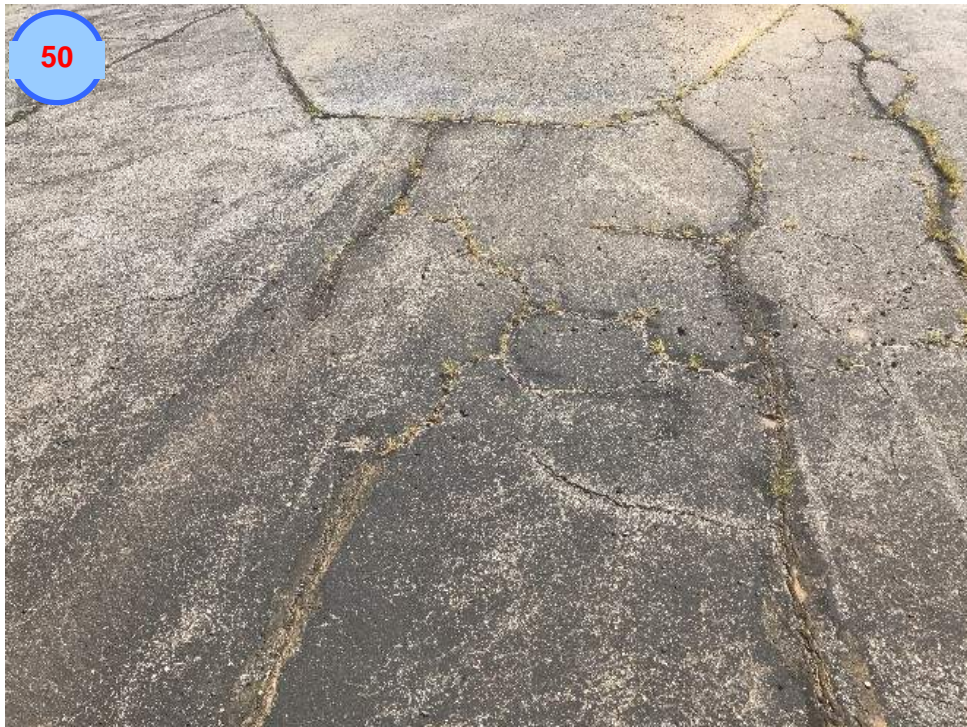
Medium Severity Weathering, Longitudinal Cracking, and Alligator Cracking East Apron
