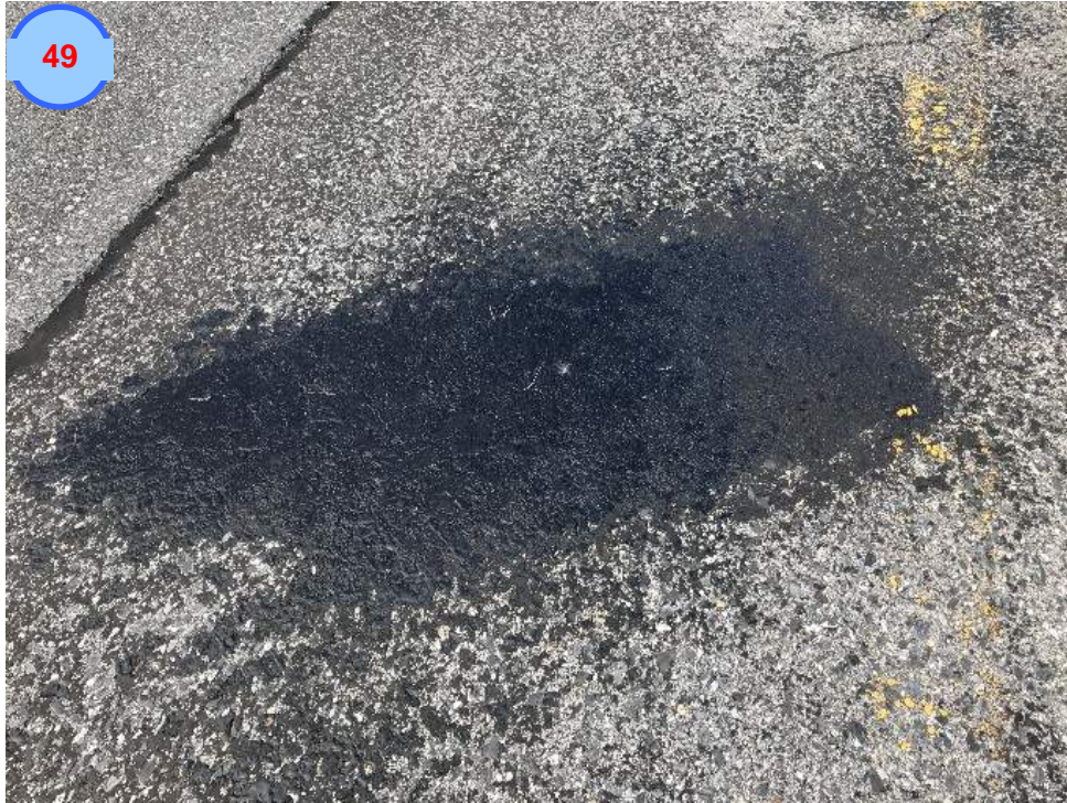
Medium Severity Bleeding and Weathering East Apron
