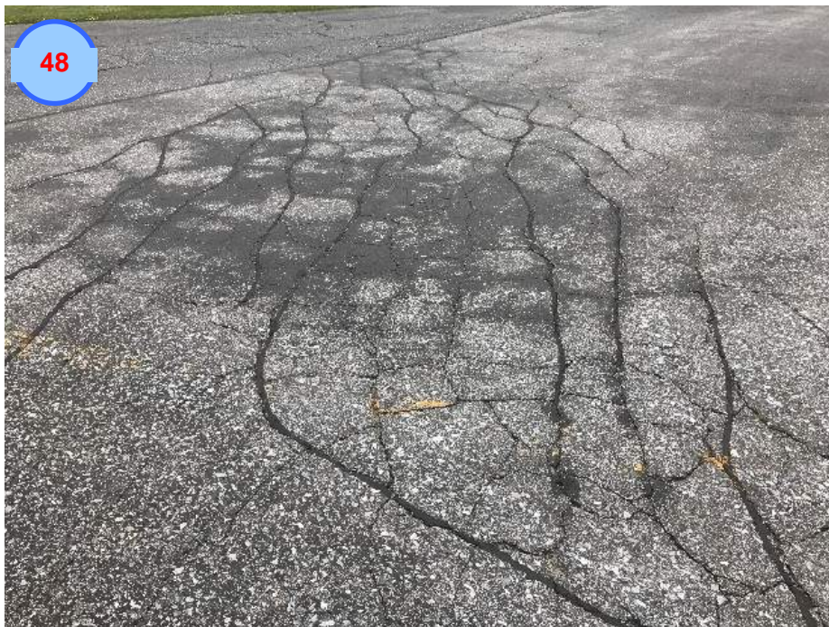
Medium Severity Alligator Cracking, Bleeding, Weathering, and Slippage Cracking
