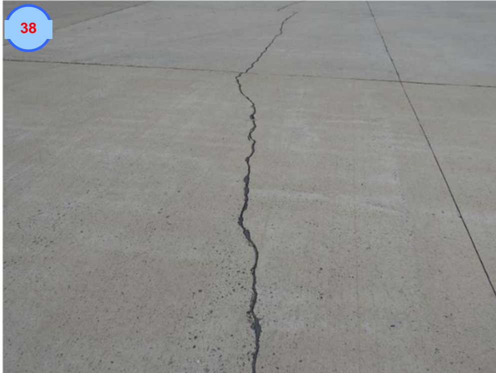
Linear Cracking Northern
