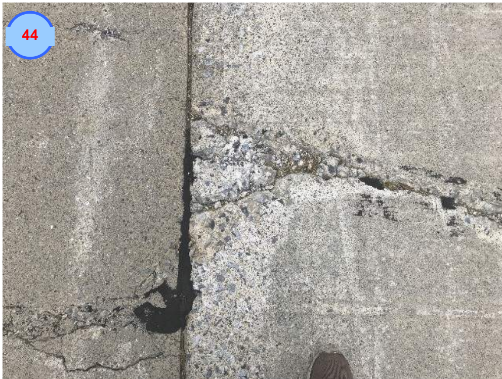
Joint Seal Damage and Spalling
