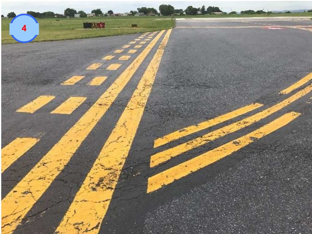
Low Severity Alligator Cracking
