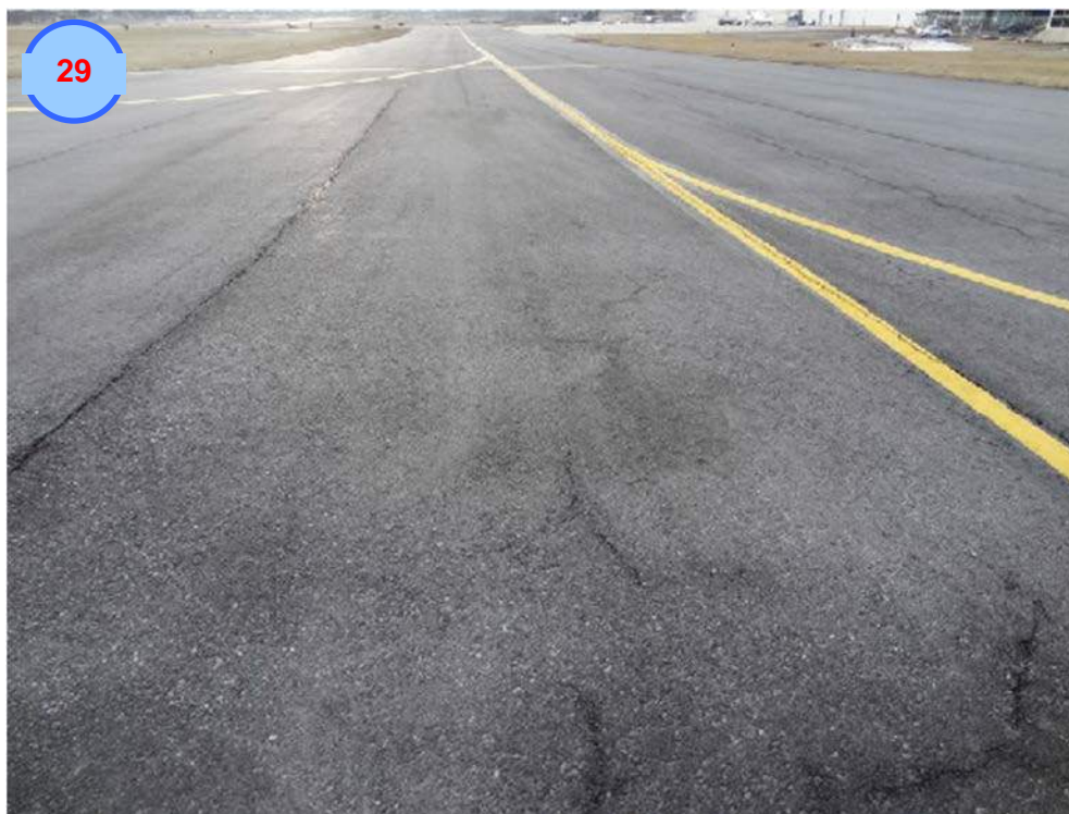
Weathering and Alligator Cracking
