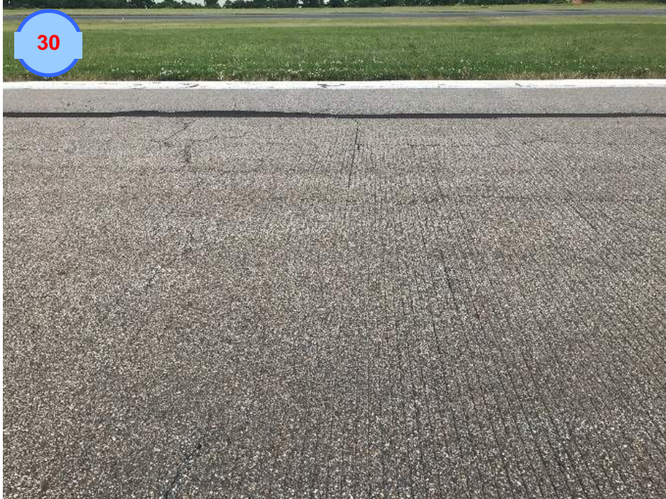
Alligator Cracking, Weathering, and Longitudinal Cracking
