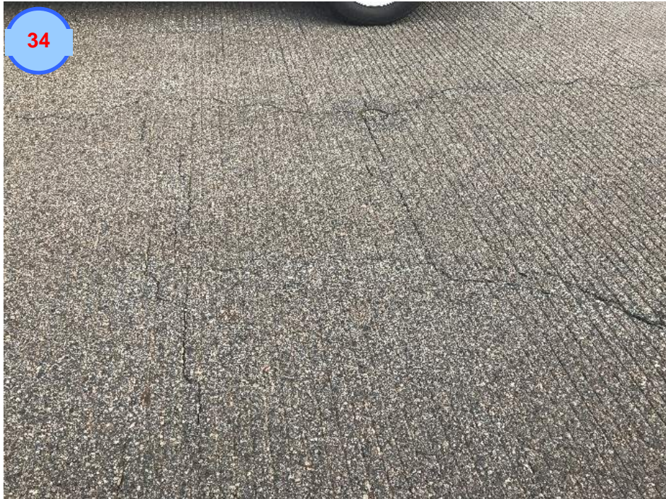
Low severity Longitudinal Cracking and Weathering
