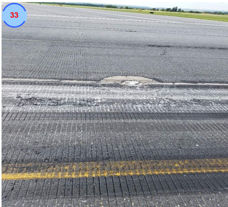
Low severity Weathering, Raveling, and Longitudinal Cracking
