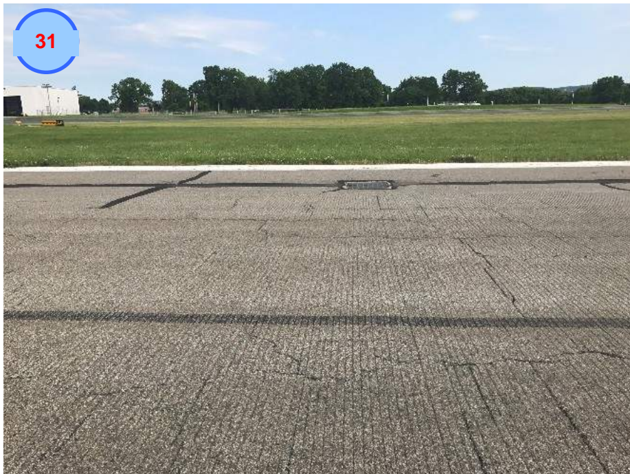
Medium Severity Block Cracking, Alligator Cracking, and Weathering
