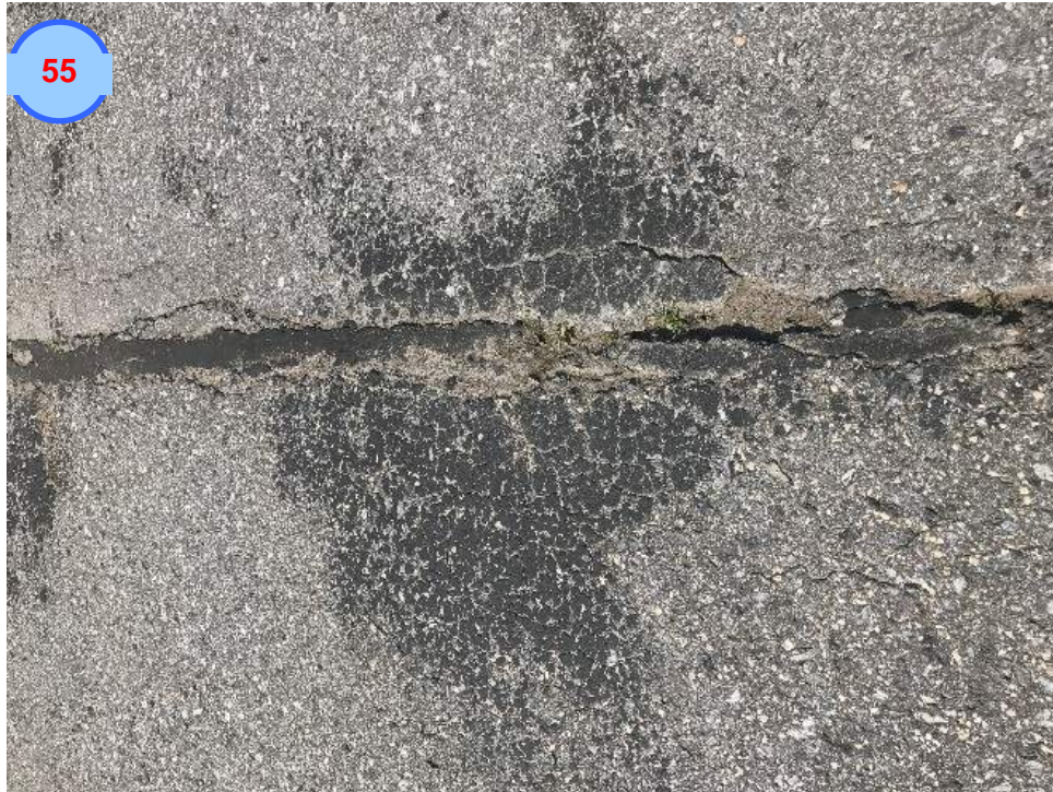
Longitudinal Cracking, Bleeding, and Weathering East Section
