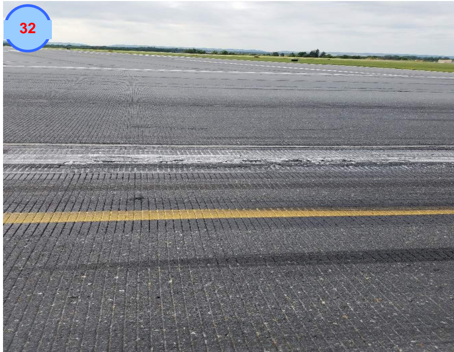
Weathering and Raveling
