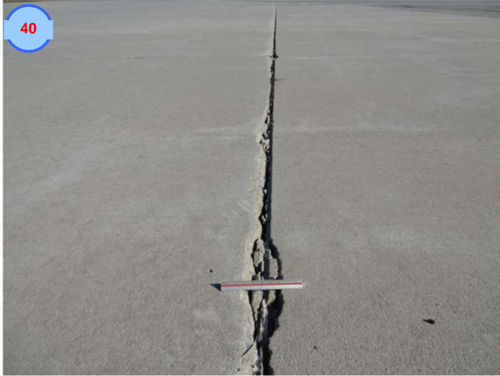
Joint Seal Damage and Joint Spalls Southwestern Portion
