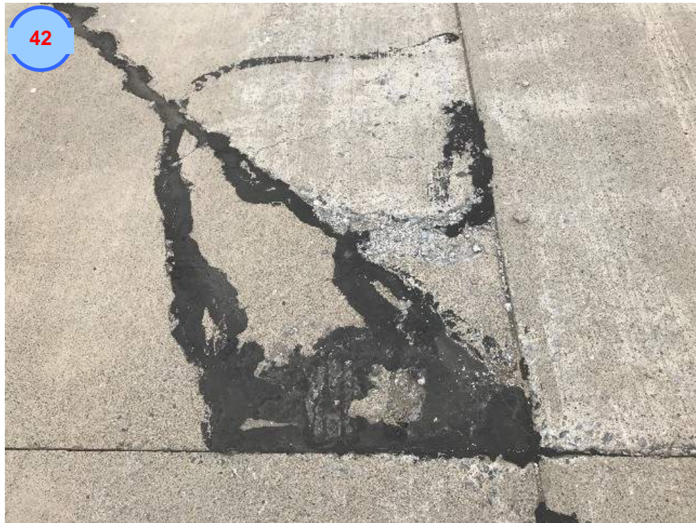
Corner Break and Joint Seal Damage
