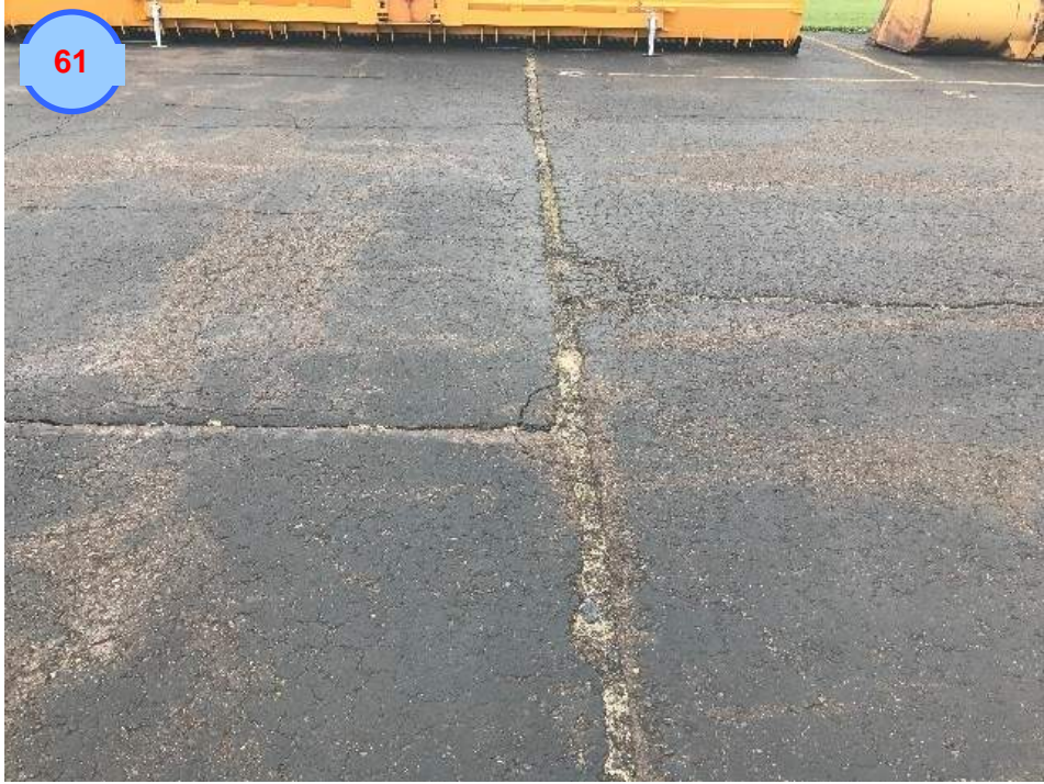
Medium Severity Joint Reflection Cracking
