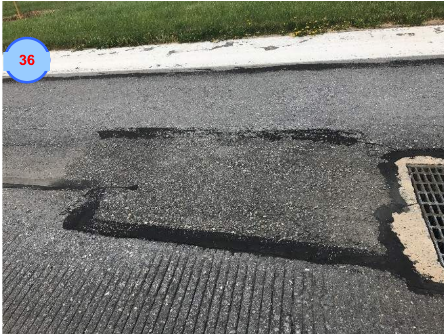
Patching, Weathering, and Raveling
