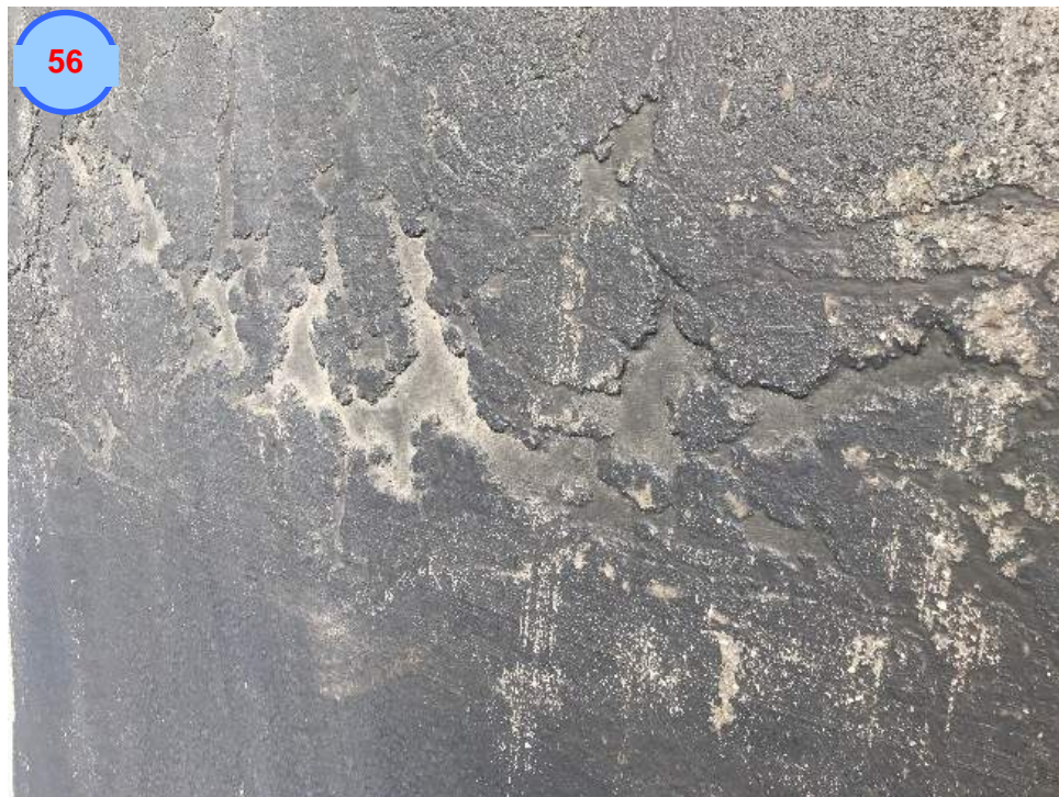
Weathering and Raveling East section
