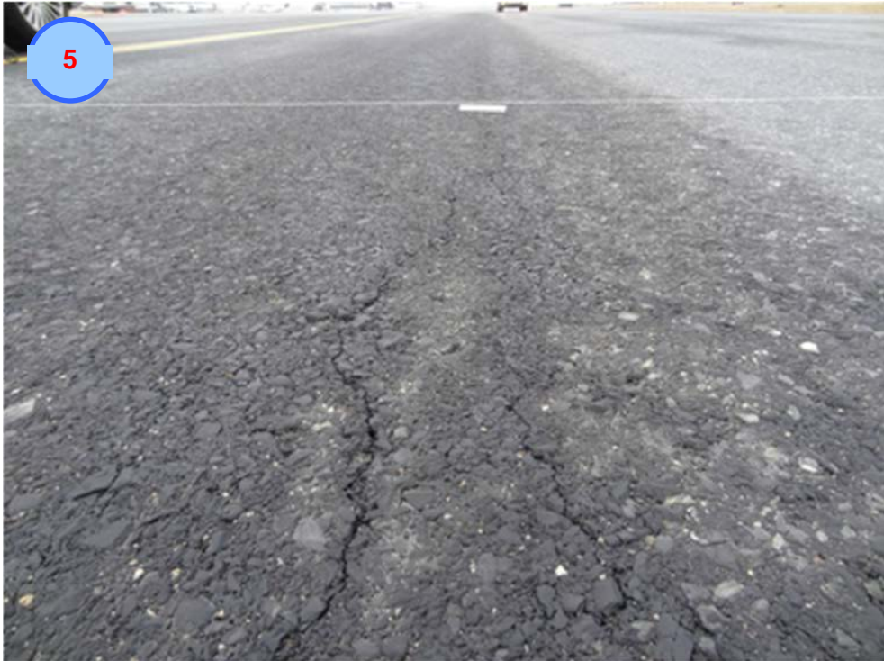
Medium Severity Weathering and Cracking
