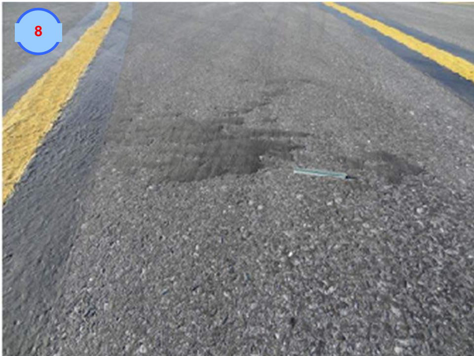
Weathering and Bleeding Taxiway A
