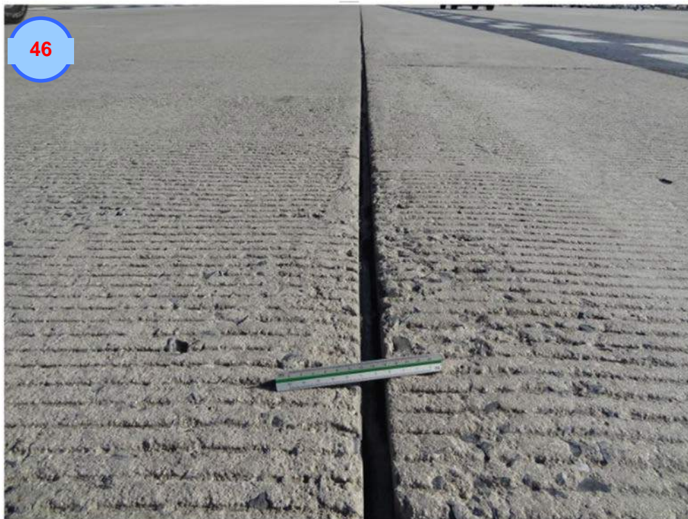
Joint Seal Damage PCC Section
