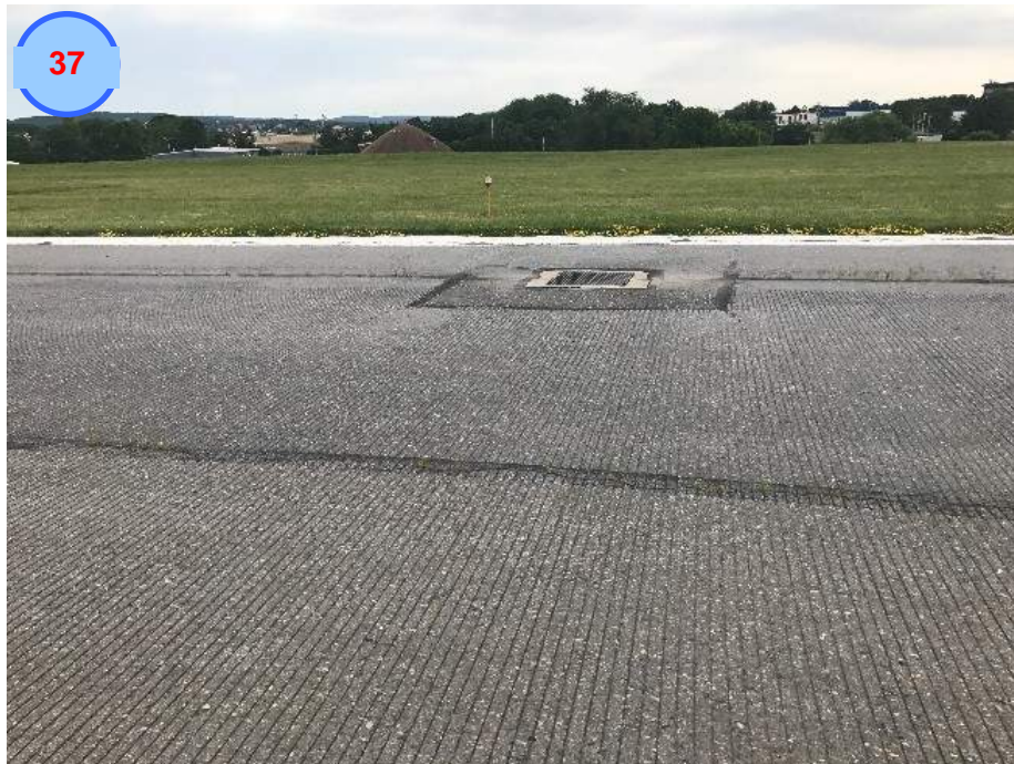
Patching, Weathering, and Longitudinal Cracking
