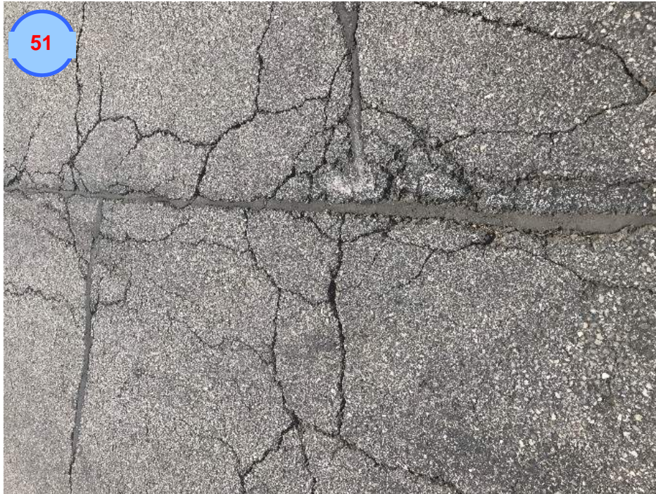
Medium Severity Alligator Cracking
