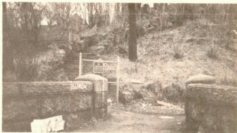
DOHERTY PARK will be the recipient of a $291,000 grant from the Federal Urban Self-Help Fund to address the deterioration of the north slope of the park.
