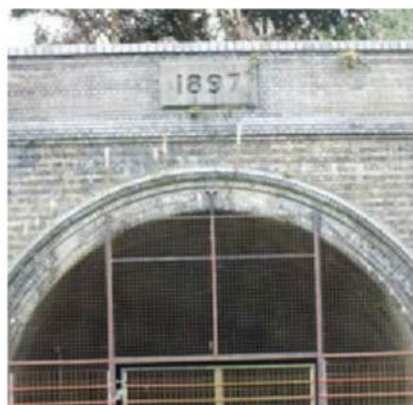
The heritage of the railway tunnel at Catesby – and the condition of the facility as a 21st-century test facility, is testament to the engineers and men who built it over a century ago but also to the specialised outlook of the UK motorsport industry
