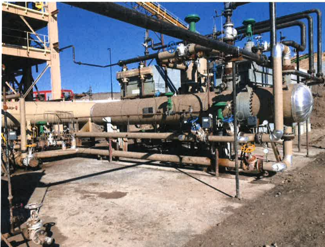
Vapour recovery system with shell and tube exchanger to heat pre-oil and flash light ends
