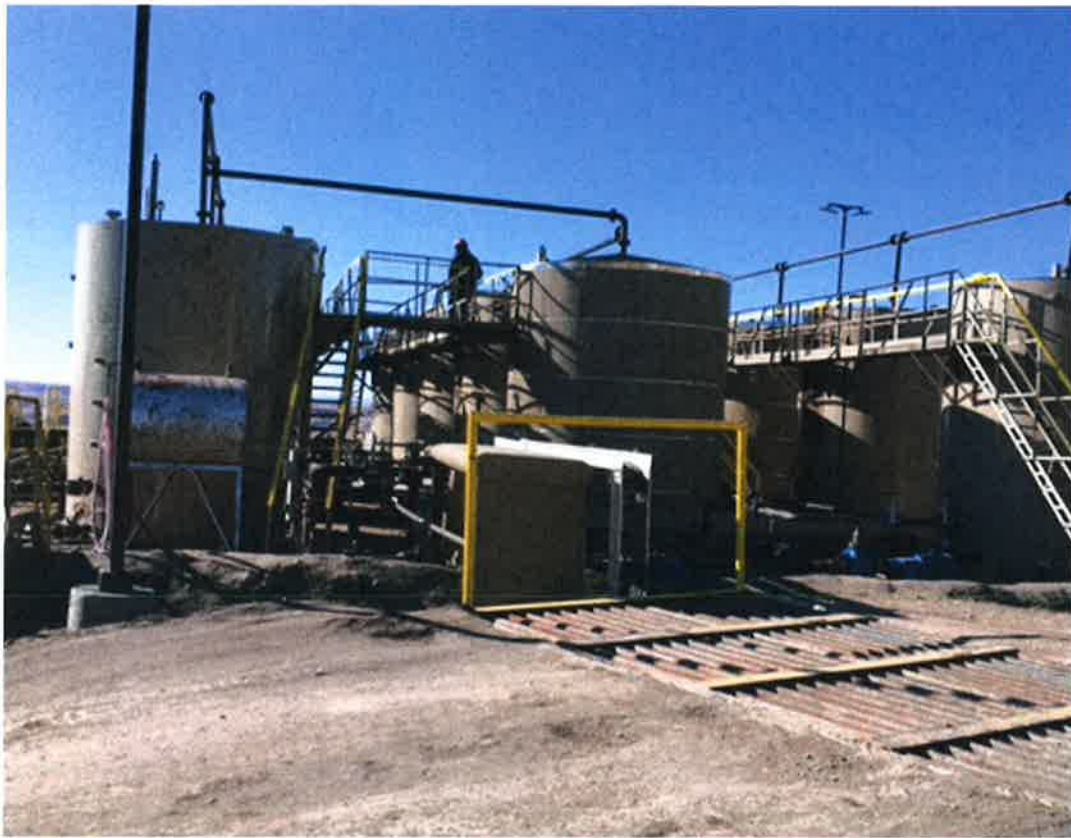
Tank farm. Sales oil on left, pre-oil in middle, slop tanks in right
