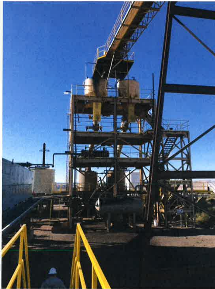
Top hopper with solvent/ore mixing tanks below
