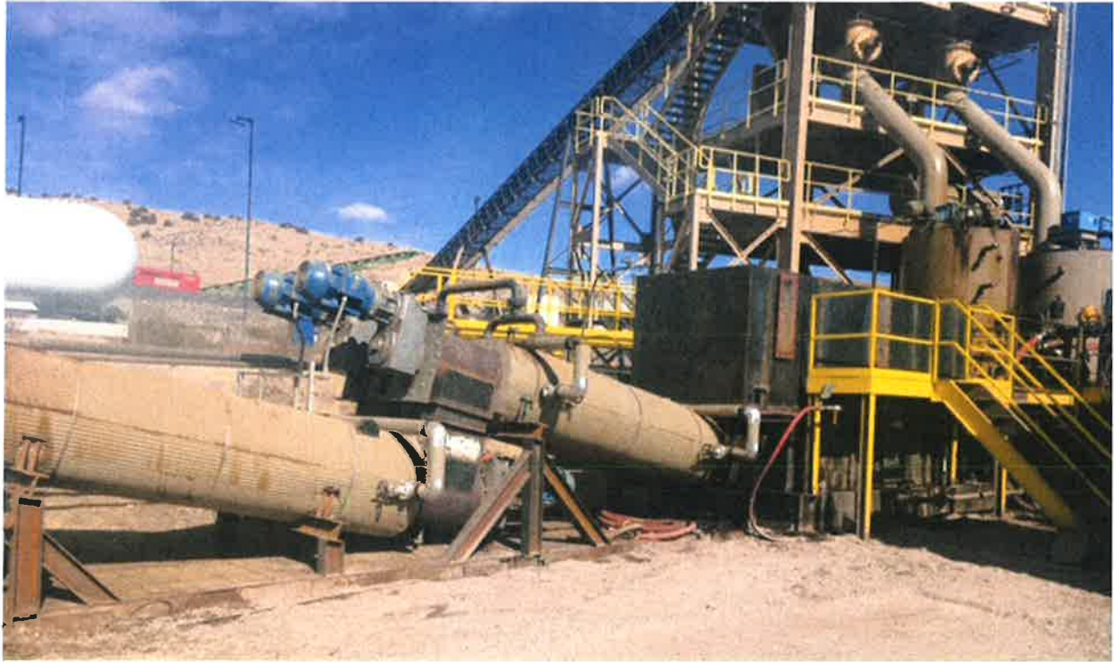
Shaker and heated auger downstream of mixing tanks
