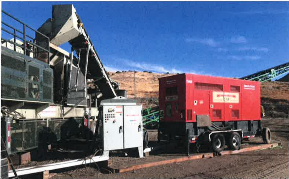
Electricity generator for Crusher
