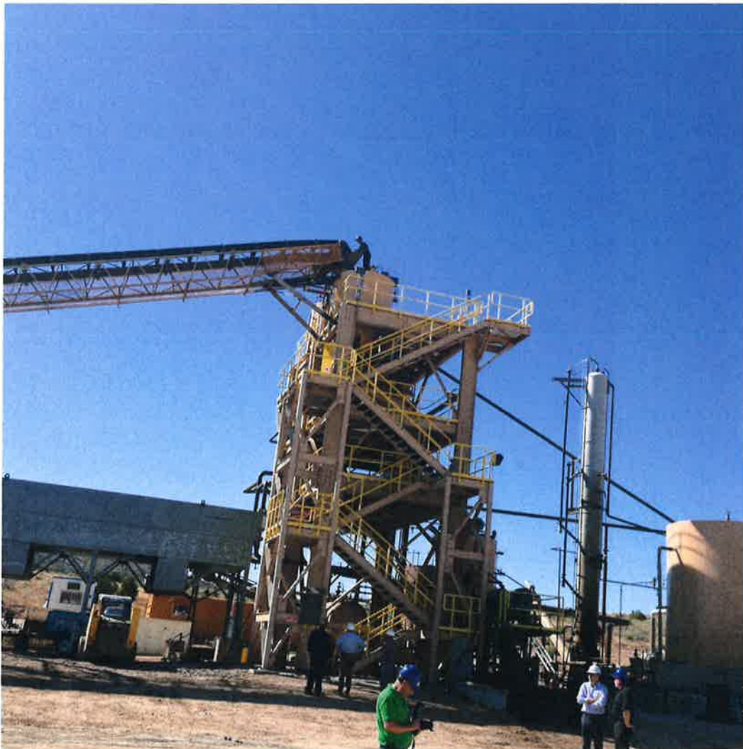
Pilot Bitumen Extraction Plant – Plant in Operation
