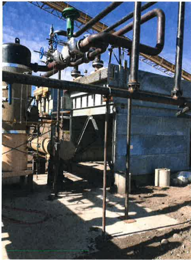
Coolers for recovery of light ends including solvent
