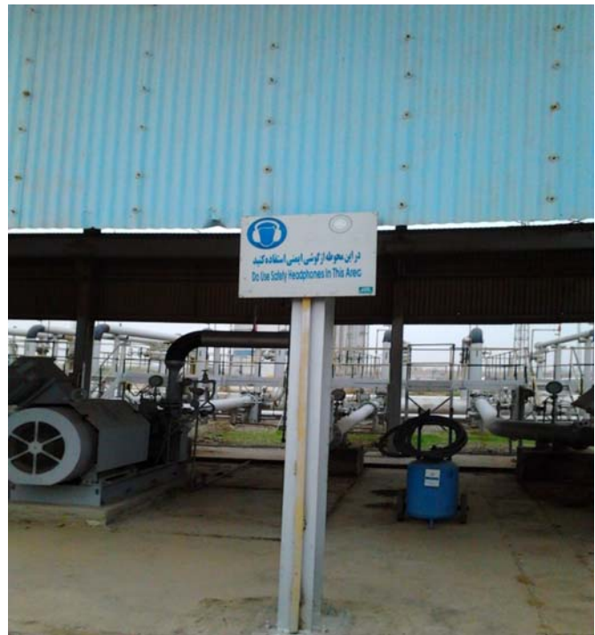
The area of air compressors in desalination factory
