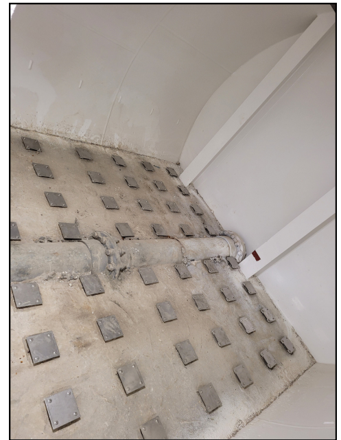
The inside of one of the pressure filters at the City's Water Treatment Plant is shown with the filter media removed.
