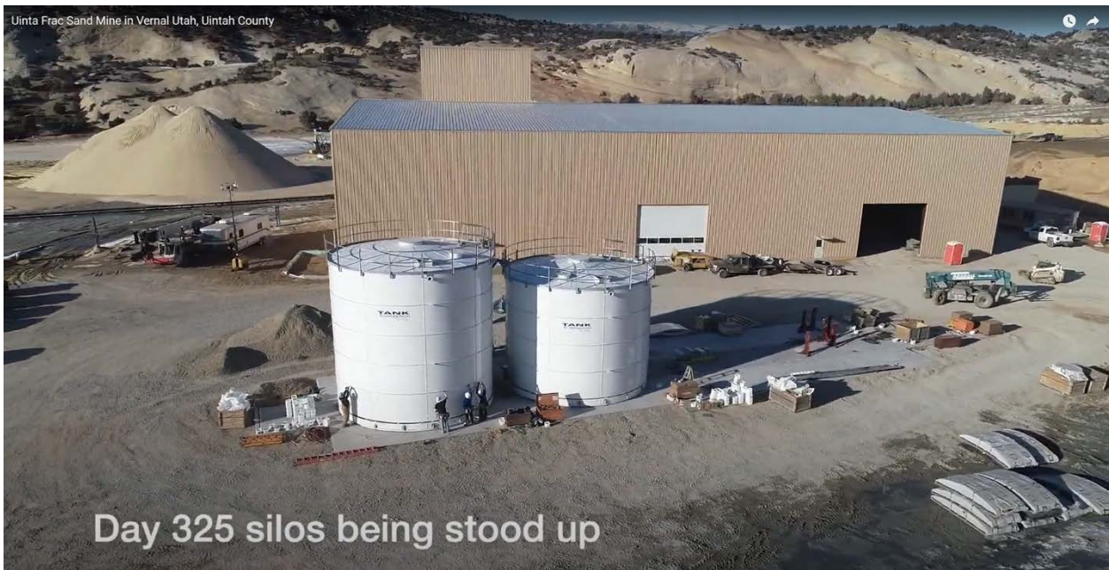
Figure 5 - Fully enclosed processing plant at the RHEX frac sand plant in Vernal, UT.
