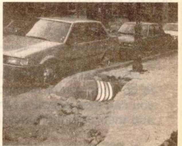
DANGEROUS HOLE on the sidewalk at 55 Main Street at the corner of Winthrop Street.
