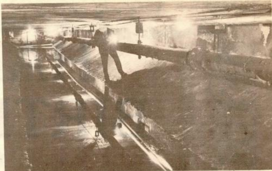
RARE VIEW - In a setting never viewed by the general public, an inspector of McCourt Cable Systems, Inc., checks his company's work beneath the roadway of the Sumner Tunnel deep below Boston Harbor. The newly installed conduits, upper right and reflected in the sump water, are an initial link in Boston's historic 210-channel cable television system which is now entering
