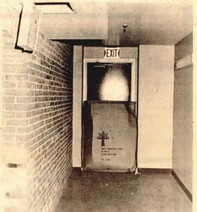
STOPPING DRAFTS: A cardboard box is placed in front of a door. Behind the box was snow which drifted in because of the space between the door and the door jamb.
