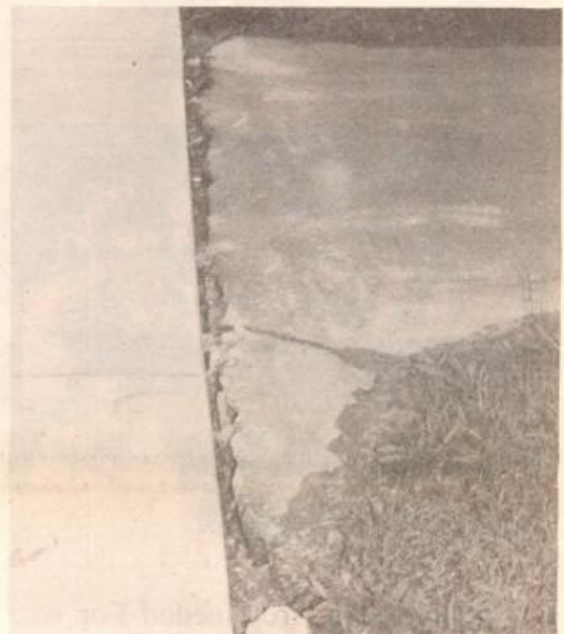
OLD RUTHERFORD AVENUE driveway at the elderly housing complex has a new sidewalk that does not quite meet the paved driveway. This condition leaves dangerous ground openings for elderly residents to maneuver with canes, walkers or in wheelchairs. (photo by Kathy Giordano)
