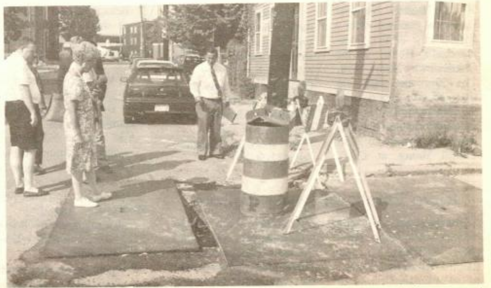
OPEN PLATES on the roadway at Lawrence and Union streets were left by the Boston Gas Co. This created a hazardous condition and tired residents who could not sleep due to the noise created when vehicles drove
