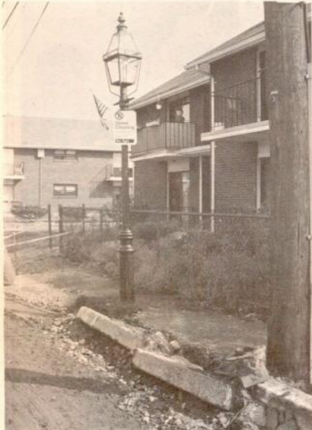
LYNDEBORO STREET curbing was left hanging onto the unpaved street. Walking and driving in that area has been hazardous for over two weeks. (photo by Kathy Giordano)
