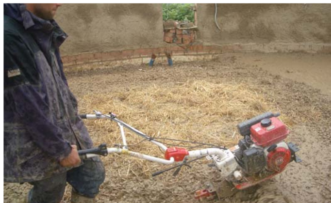
6/09: Mixing cob subfloor with a rotavator / Mezclando subsuelo de cob con rotavator
