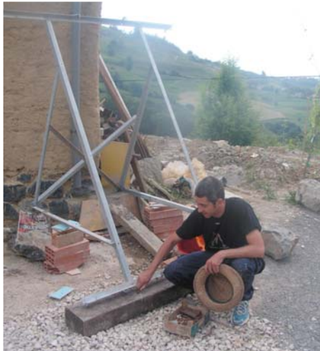
6/12: Mount for solar panels / Soporte para paneles solares
