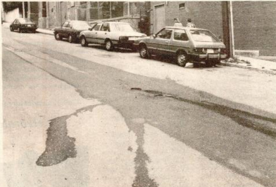
RESIDENTS have come to travel Green Street holding their noses. The leak in the street has created a waterway of sewage for almost two months. Not only is the stench unbearable, but residents utilizing the Charlestown Branch Library must cross through this waste water — some have even had their clothing soaked by the splashing from passing cars. Also, children going to the Charlestown Boys and Girls Club have been seen paddling in the puddles — some barefoot! Whatever the problem, it should be repaired — and repaired immediately. The health of the residents is at stake and two months is too long for this community to wait for this leak to be repaired. (photo by Skippy)
