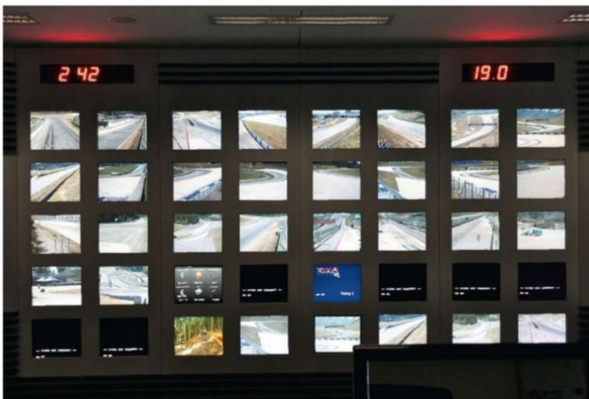
▲ The control room's 42 monitors and 26 cameras give an uninterrupted view of the entire circuit
