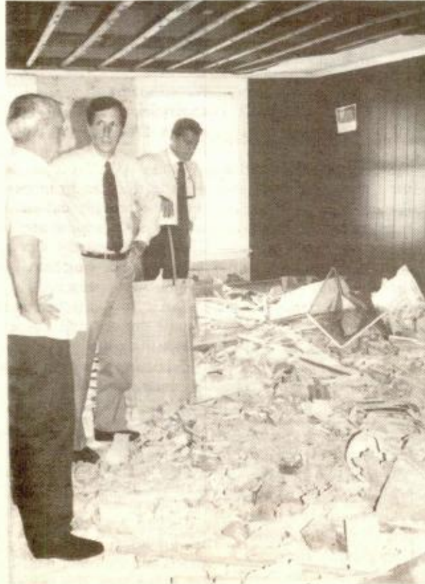
INSIDE 43 BELMONT ST., next-door neighbor John Hart (left), Inspectional Services Department Executive Director Peter Welsh and City Councillor Robert Travaglini survey the first-floor mess. The three-story abandoned house has remained virtually in the same dangerous condition for at least six months. (photo by Kathy Giordano)
