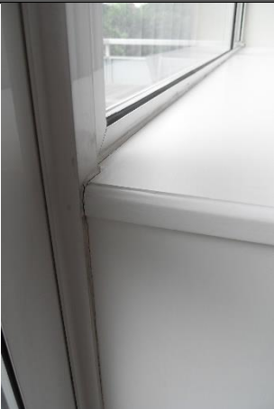
CRACKS TO WINDOW SILL
