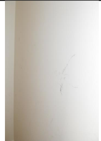
MARKS ON WALL
