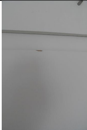
WARDROBE DOOR CHIPPED
