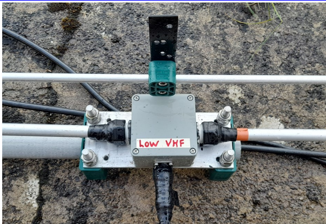
Fig. 1 Aluminium Mounting Plate and ABS Box at the Centre of the Dipole
