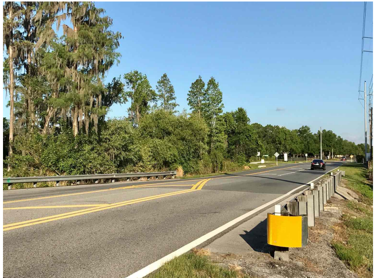
Figure 1: Area of Highest Mortality at Existing Pipe Culvert
