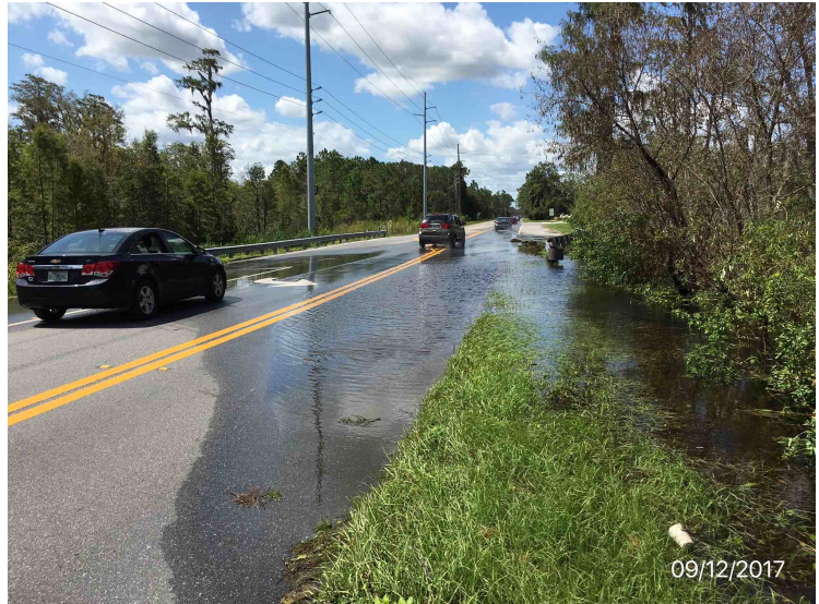
Figure 5: Hurricane Irma Flooding Reams Road Pipe Culvert
