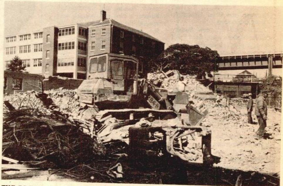
THE PRIMARY ACCESS POINT to the new development area of the Charlestown Navy Yard will be through the old Gate 4. Demolition of Building 136 was necessary to realign 5th Street with Gate 4. This new entryway will serve both automobile traffic and pedestrian access for the Charlestown community to the public park and the commercial areas of the Navy Yard.
