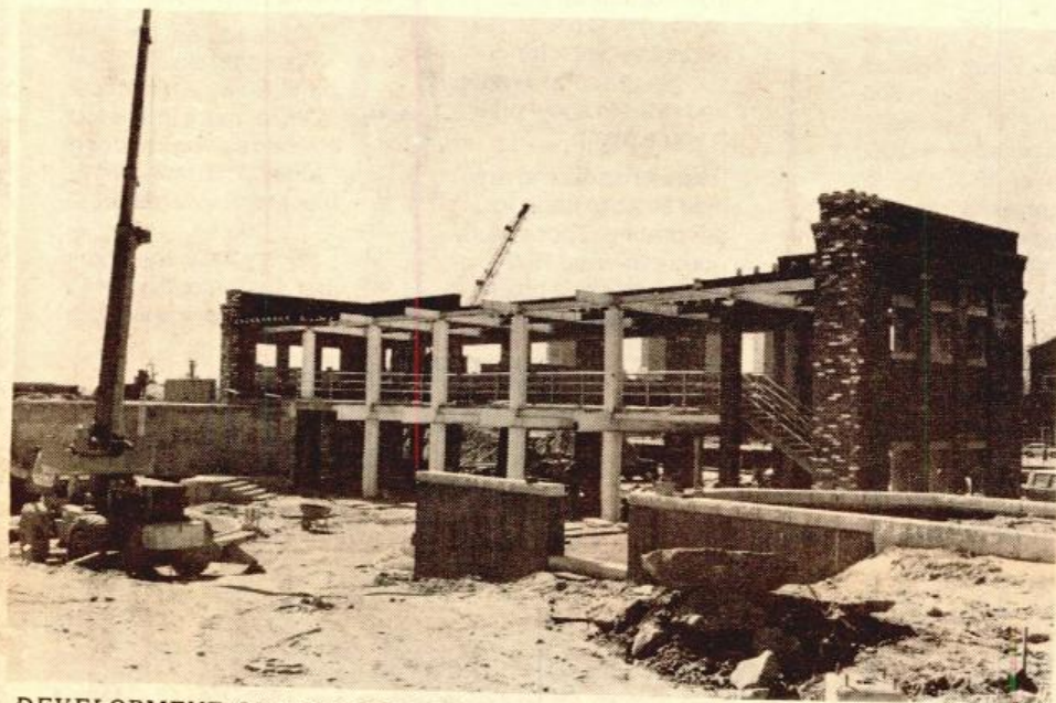
DEVELOPMENT OF SHIPYARD PARK has progressed towards its November, 1979 completion date with final landscaping and opening scheduled for next spring. This view of the pavilion area shows work being completed on the fountain and water feature in the park. The pavilion, with views of both the park and downtown Boston across the harbor, will contain a descriptive history of the Navy Yard.
