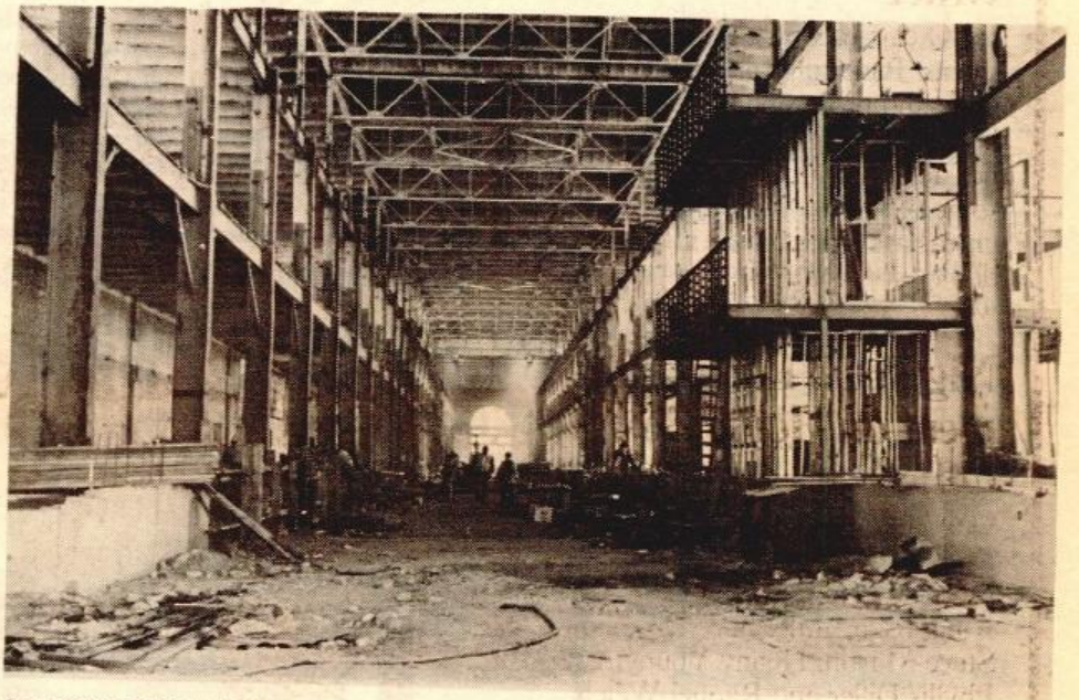
CONSTRUCTION ACTIVITY in Building 42 includes the model apartments being installed on the right above. Building 42, developed by Immobilair New England, will contain 368 units of rental housing completion is scheduled for fall 1980. This is the first phase of housing development planned by Immobilair to include 1200 units of new housing, a 500-slip marina and retail space.
