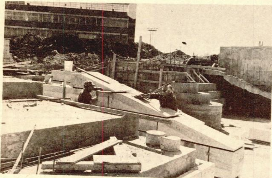
WORKERS ARE SHOWN finishing the granite stonework in the fountain area of the Shipyard Park. Designed to reflect the nautical history of the Navy Yard, the fountain will be a major feature of the 16-acre park. The park, being constructed by the Boston Redevelopment Authority, will also contain a town-pier and 50-slip marina.
