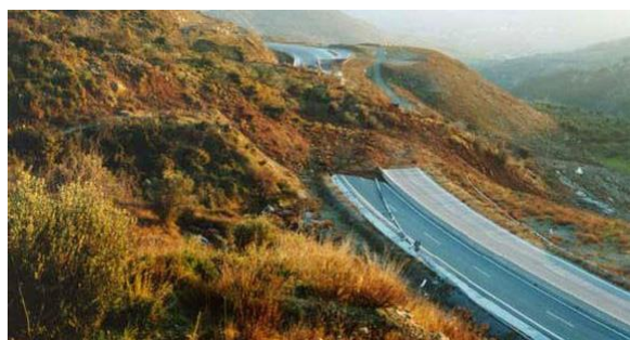
Figure 1. The Tsakona landslide (2003)
