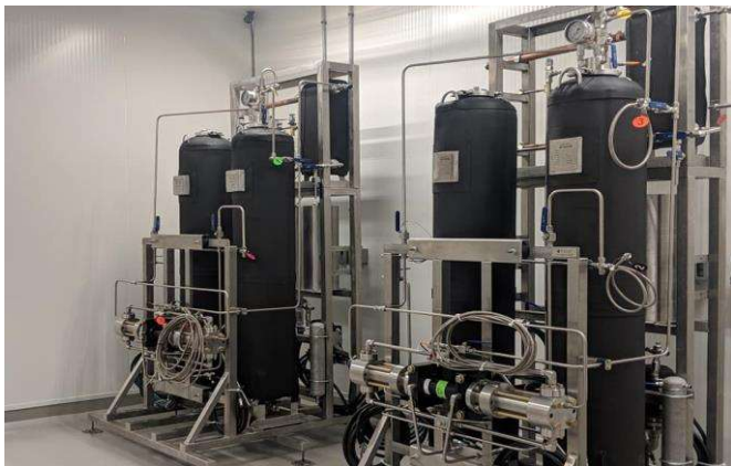
Exhibit 3: Vitalis Q90 CO 2 extraction machine at CannaCure facility
