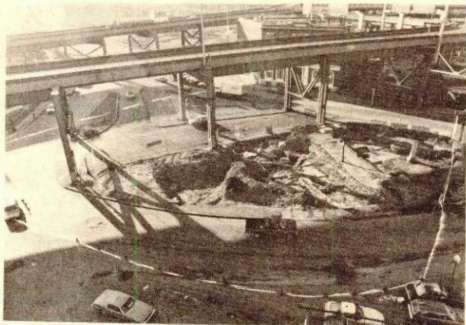
HIGHWAY CONES and white lime mark the outline of the proposed new City Square after the completion of the North Area/Central Artery project that will involve removing the
