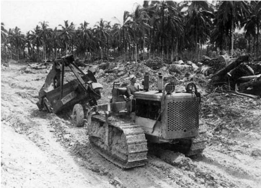
A tractor-drawn scraper of the 47th Naval Construction Battalion of Acorn 7 ripping out the airstrip at Segi from Harold Markham's coconut plantation. Some of the mature palms that made his operation profitable can be seen still standing in the background. Markham, along with other small, independent planters, was ruined by the war since the British government declined to make any compensation for war losses. He died in Sydney in 1954. (Signal Corps)
