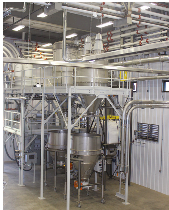
PHOTO: COPERION K-TRON
