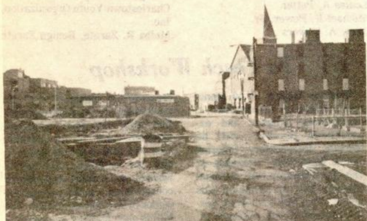
OPEN EXCAVATIONS across from a school playground poses constant danger to residents and motorists. (photo by Bill Winder)
