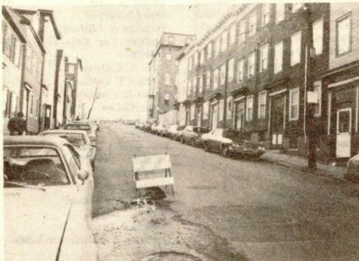
WATER LEAK and resulting pothole has plagued Lexington Street residents. (photo by Bill Winder)
