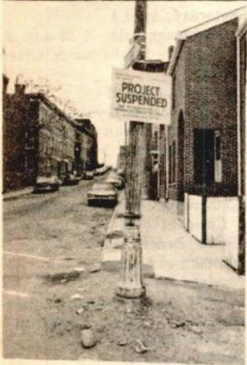
PROJECT SUSPENDED signs posted on many Charlestown streets. Residents seek answers as to when these many projects will resume as present conditions are dangerous to the persons and property of residents. (photo by Bill Winder)
