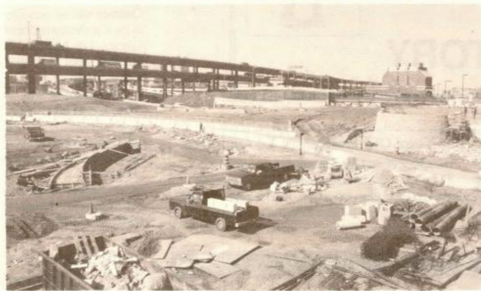
WORK IS PROGRESSING on the new Paul Revere Landing Park, adjacent to the North Washington Street Bridge. (photo by Ken Stone)
