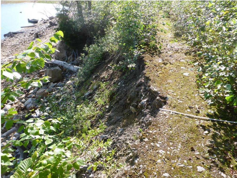
Photo 9. View east along the existing access road where sloughing is present
