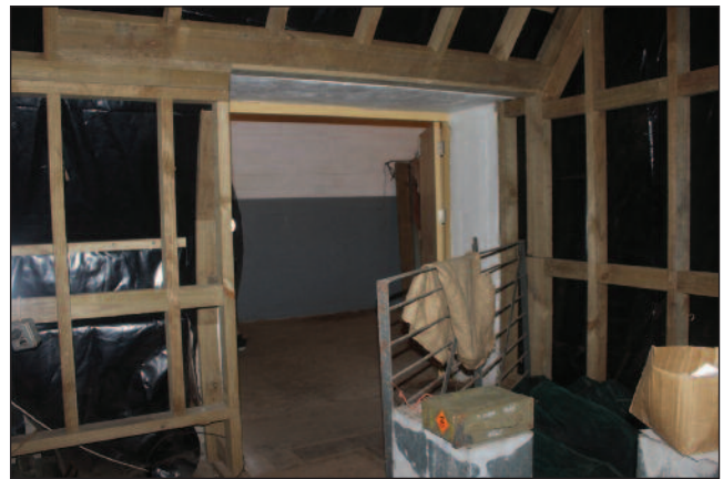
its anteroom. It was later divided into two rooms. Right: The Wrights Hill Preservation Society is in the throes of its reconstruction.
