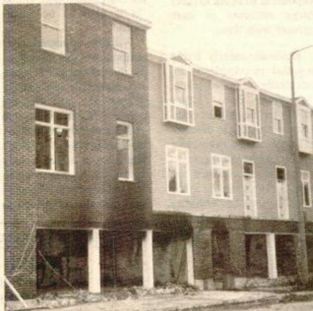
THE BOSTON FIRE DEPARTMENT responded to a fire at 430 Medford Street, the site of the construction of the new Cobblestone Landing housing, on Sunday, October 11 at 4:17 a.m. A spokesman from the Boston Fire Department stated that the fire started in the garage area under the new houses, which was being used as storage and that fire fighters were on the scene for approximately one hour. The Fire Department estimated the damage at $10,000 and attributed the cause as arson.
