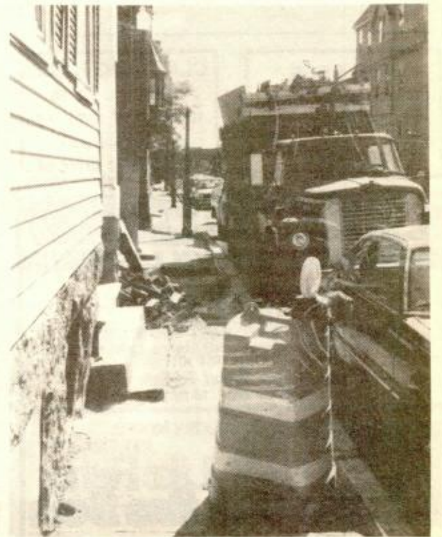
THE SIDEWALK on Warren Street, between Pleasant Street and Monument Avenue, has been an area of concern for residents. Complaints have included the fact that the sidewalk is too narrow to meet the needs of the heavy pedestrian traffic; a pile of bricks is visible, creating a hazard on the sidewalk; and a barrel covers the location where a gas lamp pole was removed despite an agreement to adjust its placement, leaving a dark area along this narrow sidewalk.
