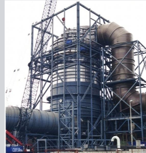
Power plant in Samrah, Jordan
