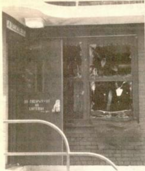
A ONE-ALARM FIRE at 74 Decatur St. early Wednesday afternoon gutted the first-floor apartment and resulted in an estimated
